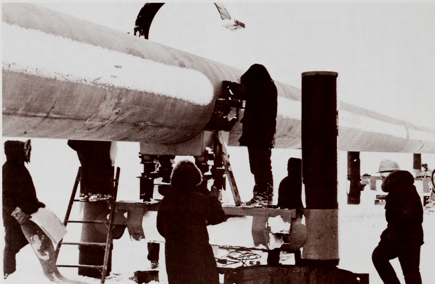
Elevated pipelines are designed to protect permafrost. (Atlantic Richfield Company)
