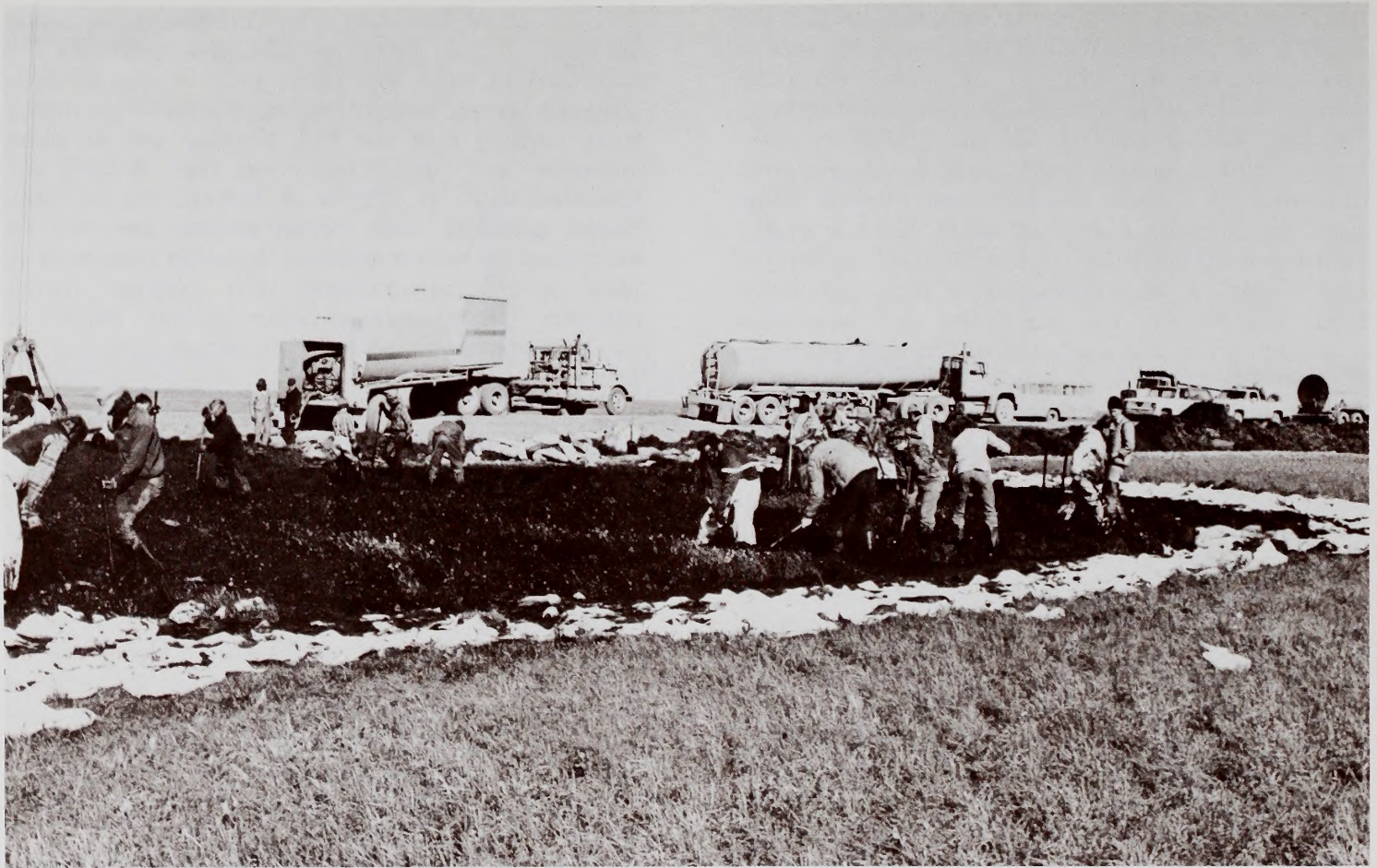
Clean-up crews used vacuum trucks, sorbent materials, water, and hand tools to remove oil spilled during an accident on the trans-Alaska pipeline. (Alyeska Pipeline Service Company)
