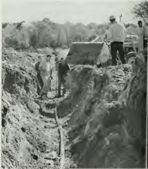
Coaxial cable in a trench on the hardened route. Trench is about to be back-filled.
