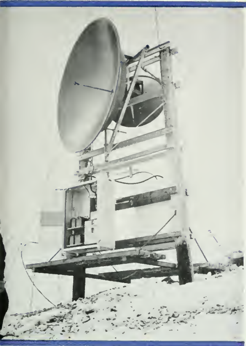
T-1 microwave repeater at Chink's Peak, Idaho. One of first installations of this system.
