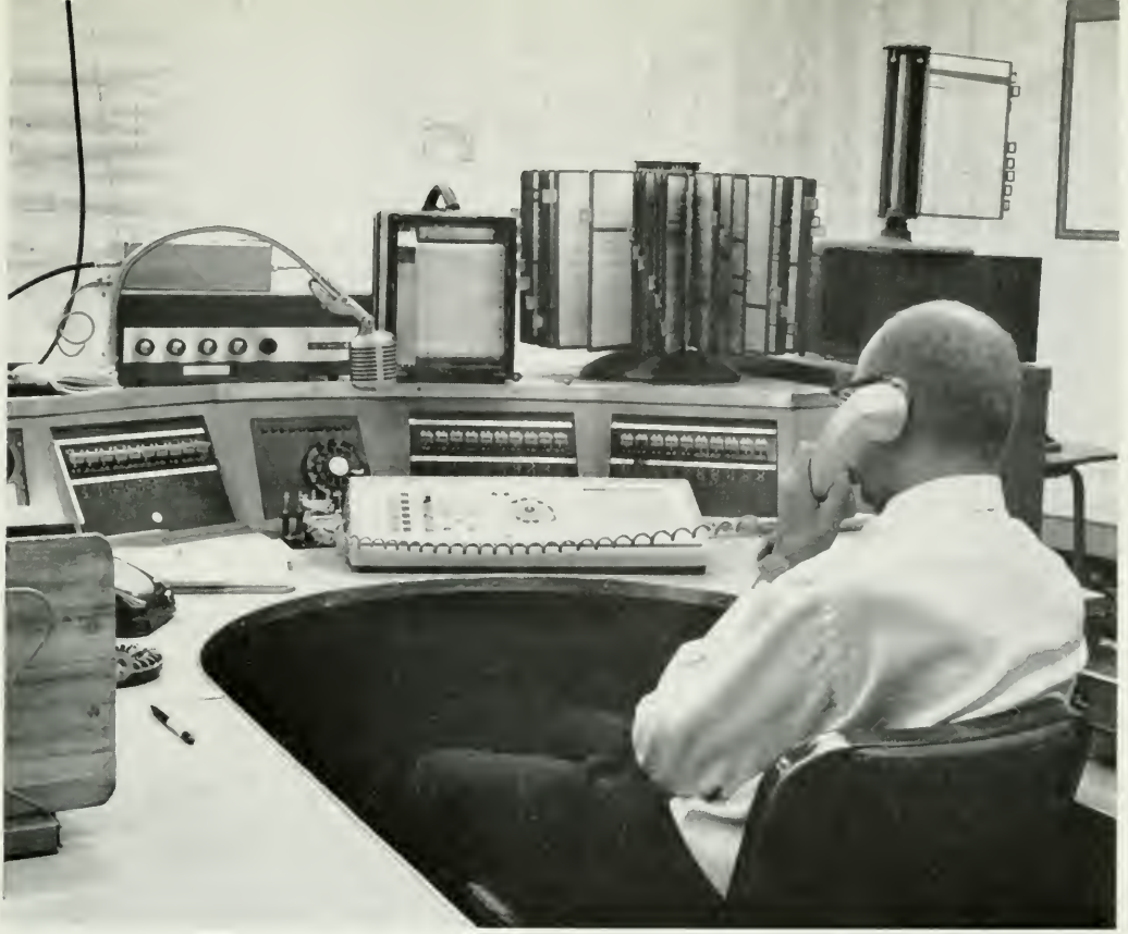
A dispatcher at the Public Service Company of Colorado uses a new desk-top switchboard, invention of Mountain States Telephone engineers, which replaces the array of complicated equipment behind it. Touch-Tone phone buttons give easy access to any of 100 lines.
