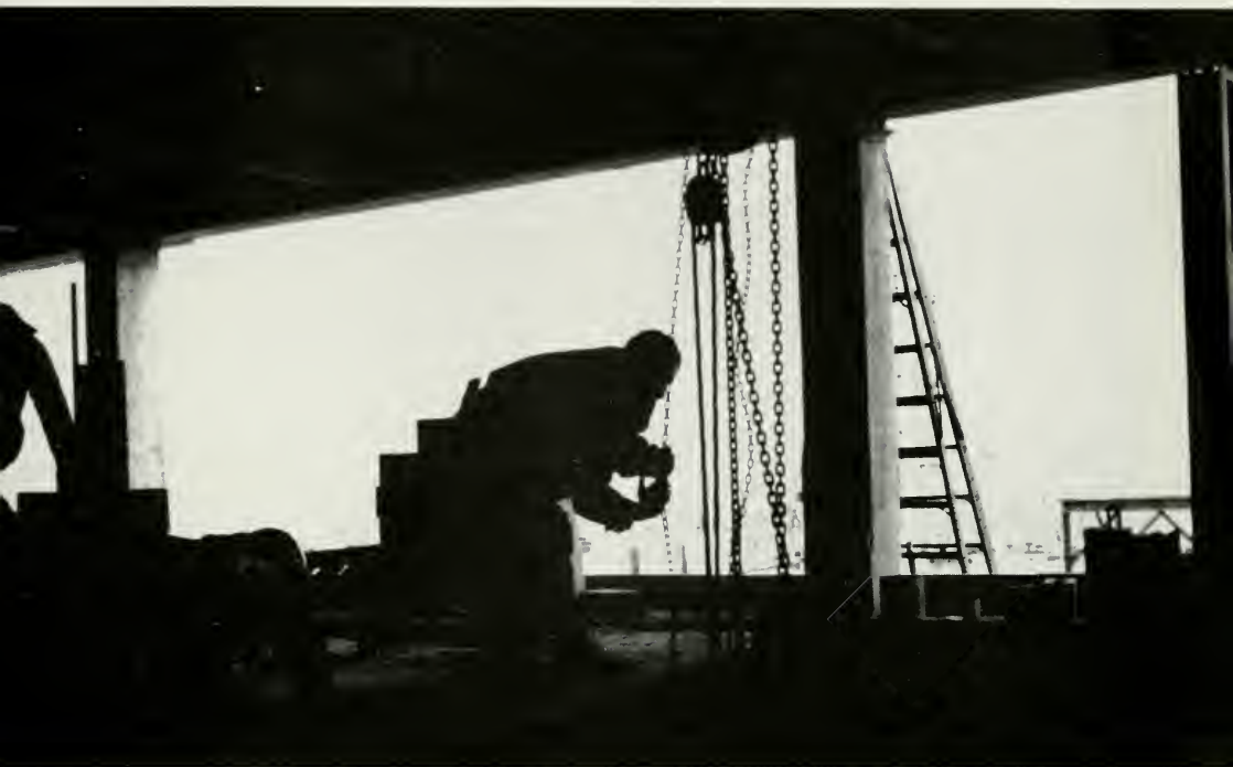
Bell System construction program provides for expanding, improving service at all levels; here, for example, extra floors are being added to an office to increase switching capacity.
