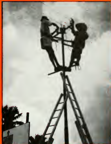
Nigerian plant men work on a telephone pole in the Eastern Region.
