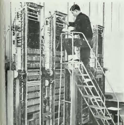
Final adjustments for one of bays of equipment in 100A Protection Switching System.
