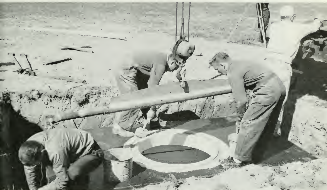
Pre-cast manholes, a recent development, assure uniform high quality construction at lowest possible cost. Above, a collar is placed on a pre-cast manhole on the new L-4 route in Ohio.
