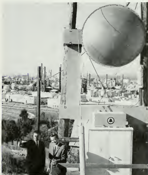
Microwave system installed by Bell System for oil company. It transmits high speed data between computers at refinery above and those at the company's headquarters.
