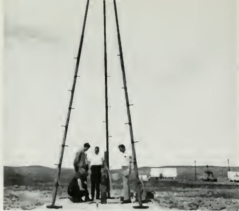
Telephone installers check Project LASA sensor before it is lowered into place.
