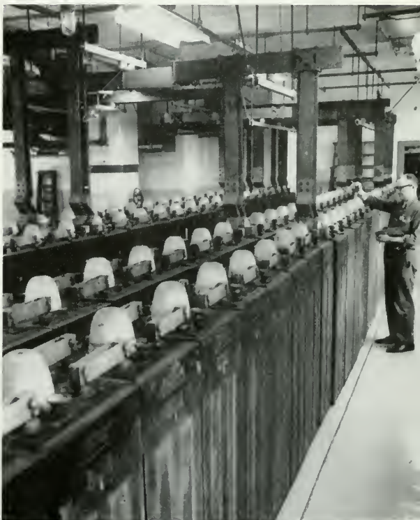
Massive batteries in Bell Telephone Company central offices provide the DC needed for transmitting, switching, receiving calls.
