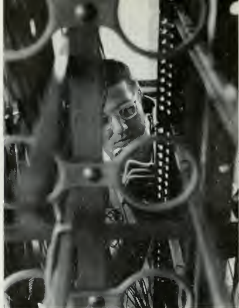
Western Electric installer tests switching equipment made by W.E. for NASA center.
