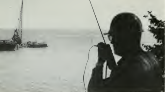
Long Lines man coordinates shore operation as armored cable is laid under Hudson River.
