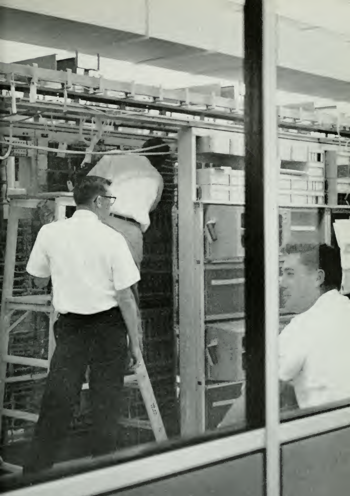
The Bell System's first commercial ESS office being installed at Succasunna by Western Electric.
