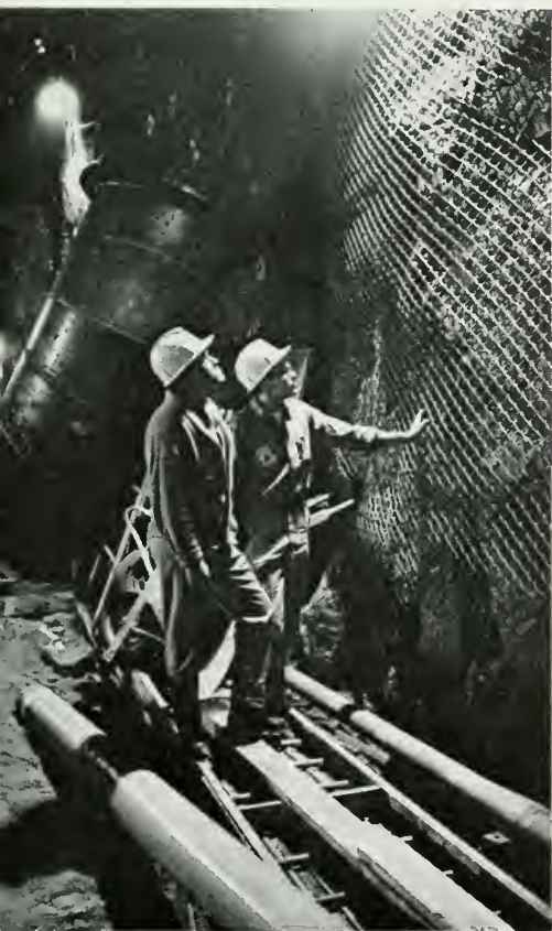
W. E. installers inside granite tunnels of NORAD center in Cheyenne Mountain.
