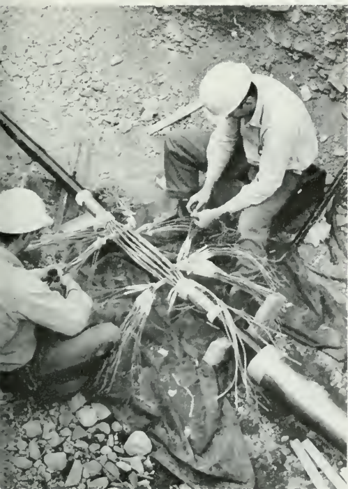
Scene above shows a coaxial cable being spliced. The cable has been laid in a deep trench in section of “hardened” route.
