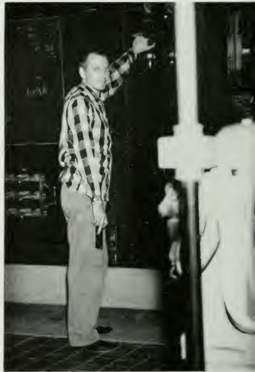
New York Telephone Company powerman switches to the emergency power which is kept on standby in all central offices.
