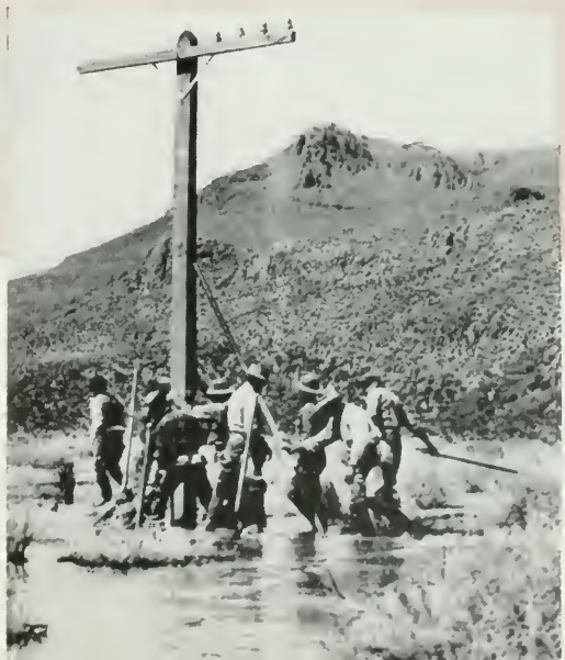
A pole rises in a salt sink. Holes were easy to dig in mud flats, but often caved in before the poles could be set.
