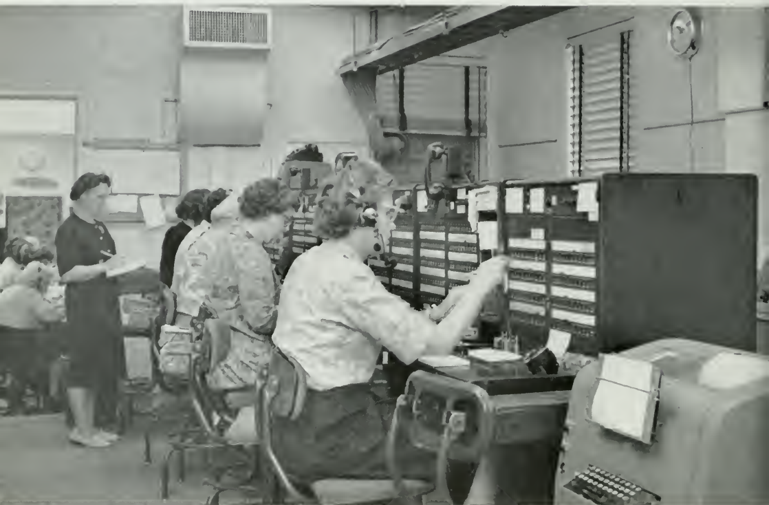
Operating room of an answering service bureau today. These switchboards function well, but the 1A Telephone Answering System will enable many bureaus to do the job more efficiently.
