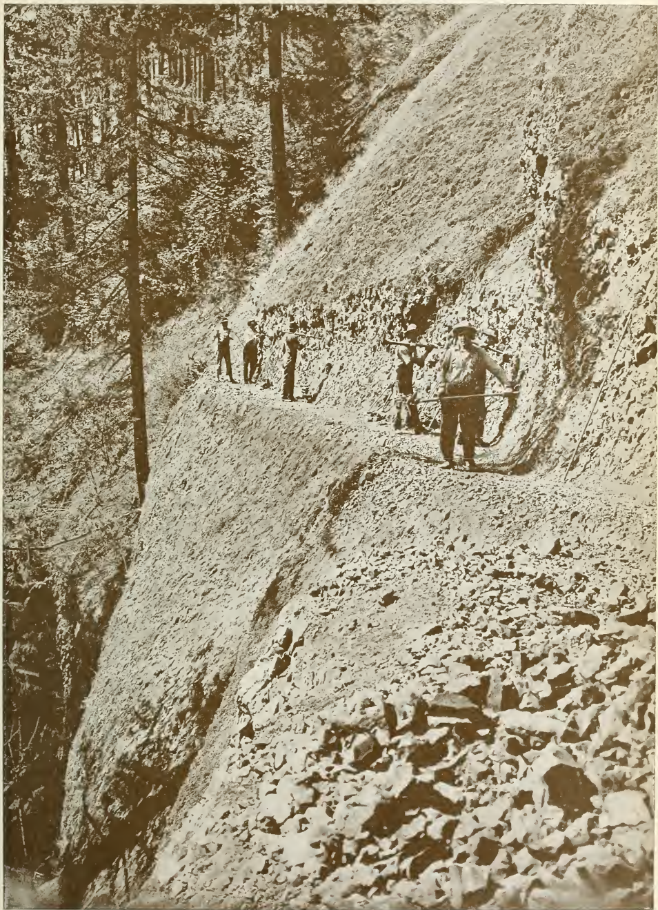
Building a Forest Service trail in a National Forest in Oregon. More than 2,600 miles of such trails have been constructed in the National Forests in the State.
