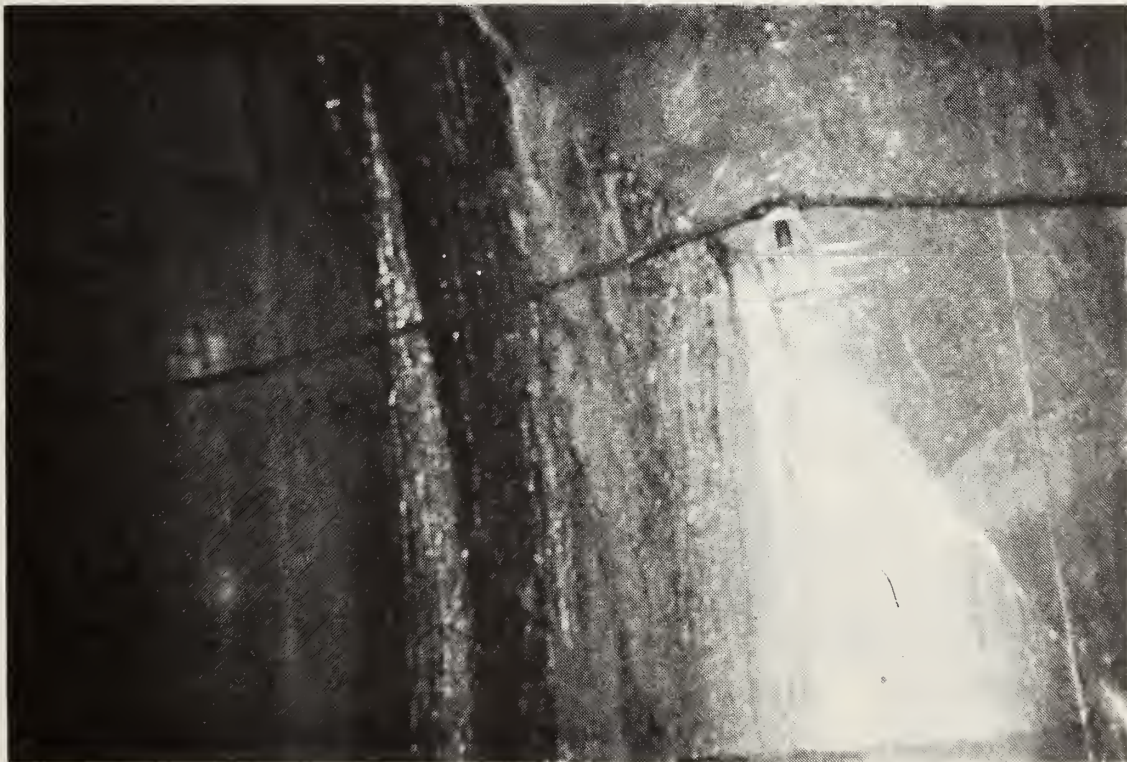
FIGURE 9.19 CALCIFICATION AND SETTLEMENTS AROUND THE CRACK AREA (ROUTE 131-A)
