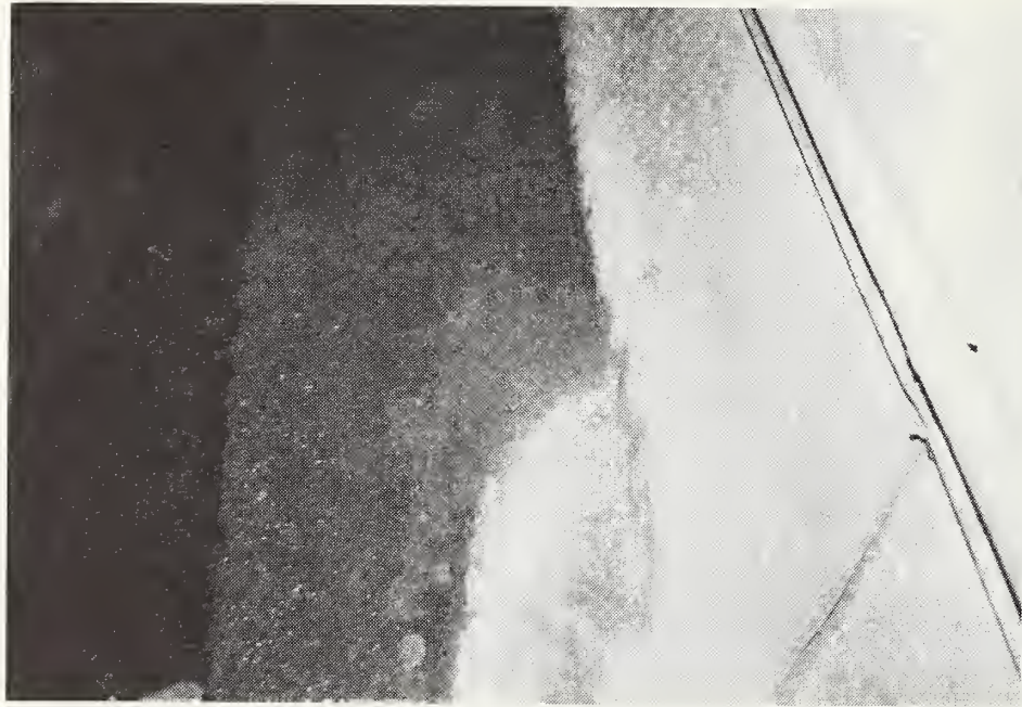
FIGURE 8.5 CALCIFICATION AND PRECIPITATIONS CAUSED BY LEAKING WATER
