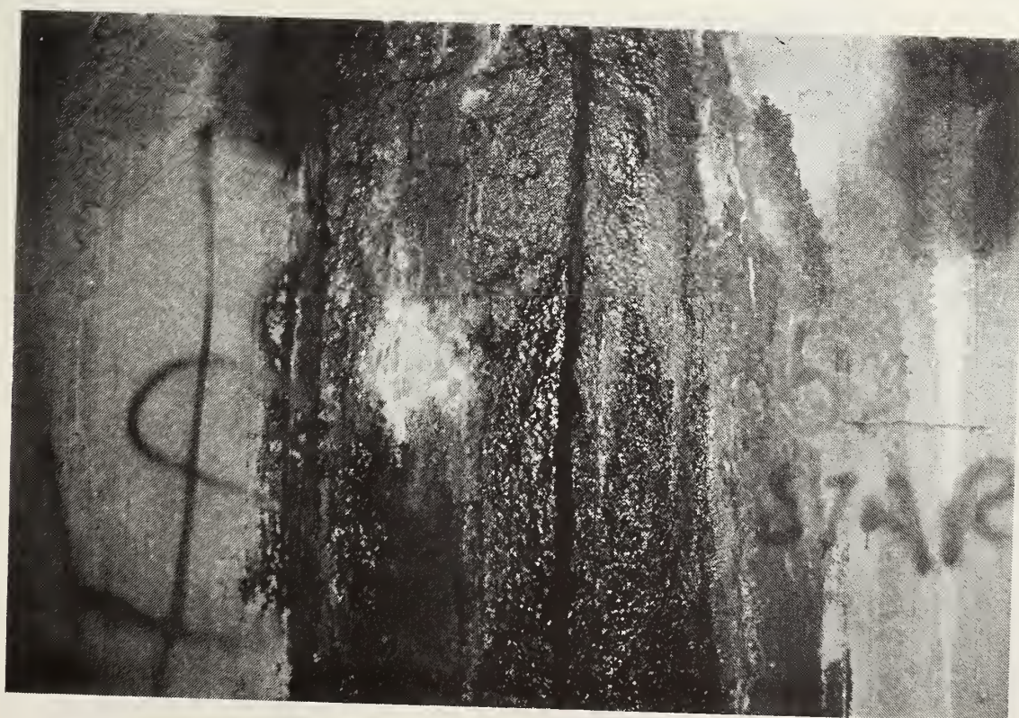
FIGURE 9.8 LEAKS THROUGH WALL JOINTS
