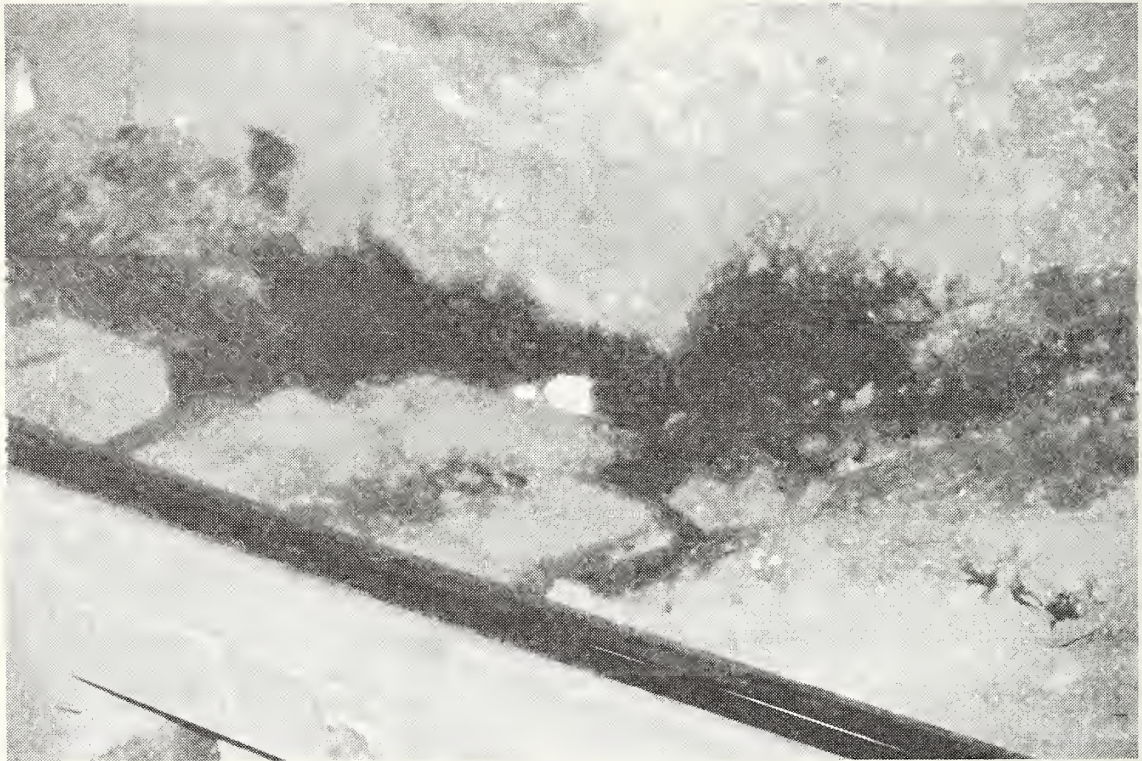
FIGURE 7.2 BALLAST WASHED OUT BY STREAMS OF RUNNING WATER (RED LINE, SOUTH STATION)
