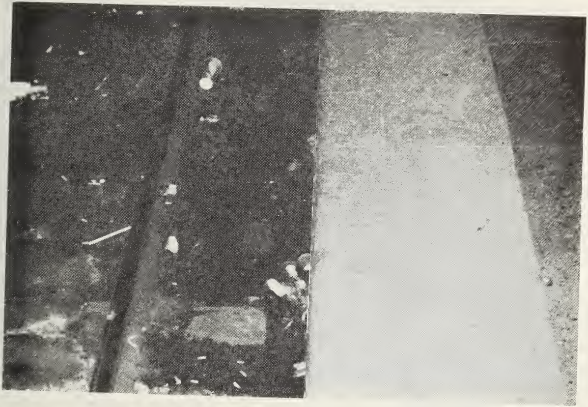
FIGURE 7.12 WATER STREAM IN TRACKBED (BLUE LINE, AQUARIUM STATION)
