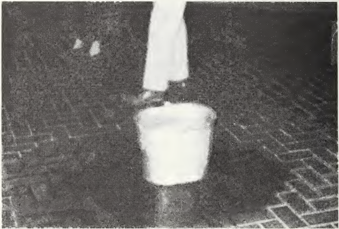
FIGURE 6.6 SAFETY HAZARD DUE TO WATER INTRUSION THROUGH STATION CEILING
