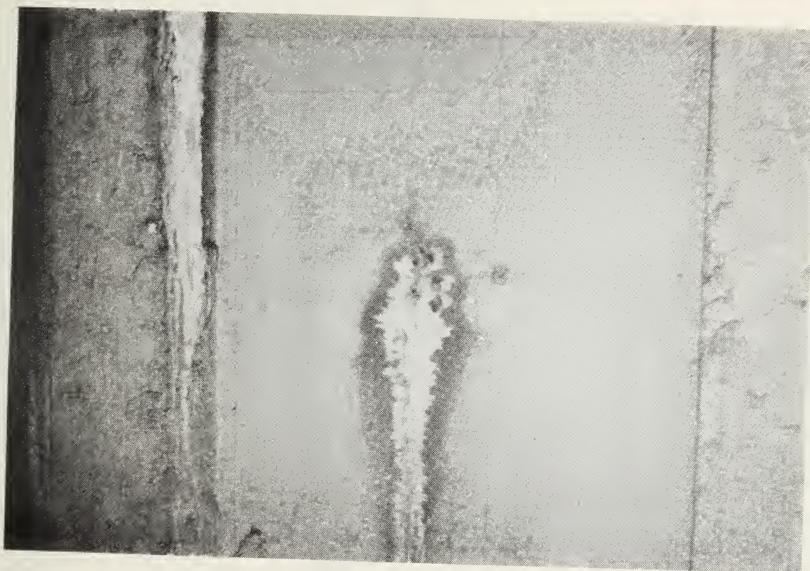
FIGURE 9.7 LEAKS THROUGH SHRINKAGE CRACKS
