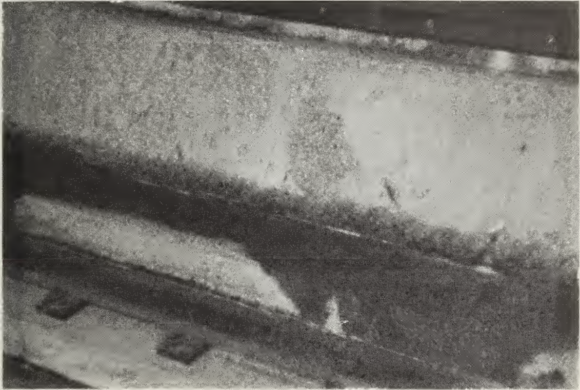
FIGURE 5.3 LEAKS ONTO TRACKBED
