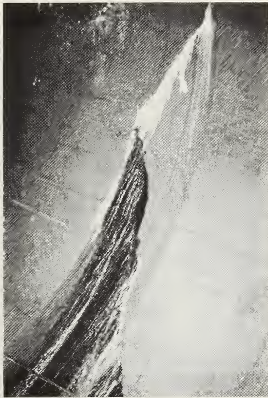
FIGURE 9.18 CALCIFICATION AROUND THE CRACKS (ROUTE 131-A)
