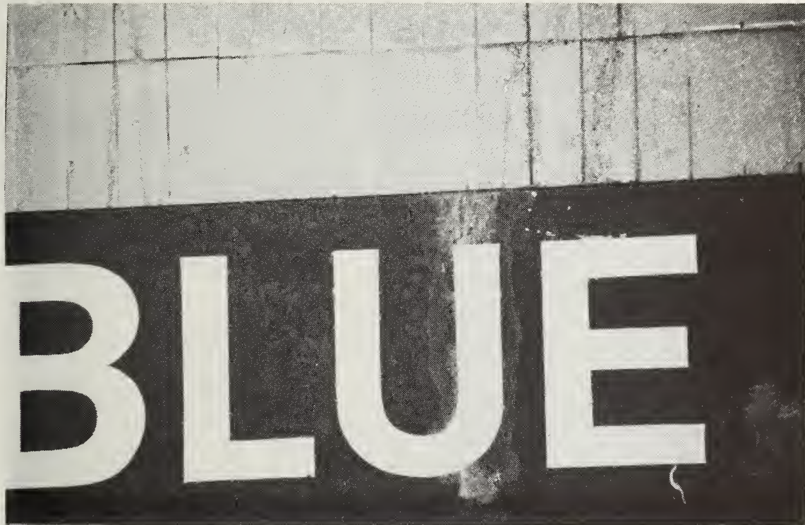
FIGURE 7.6 DETERIORATION OF PAINT (BLUE LINE, AQUARIUM STATION)
