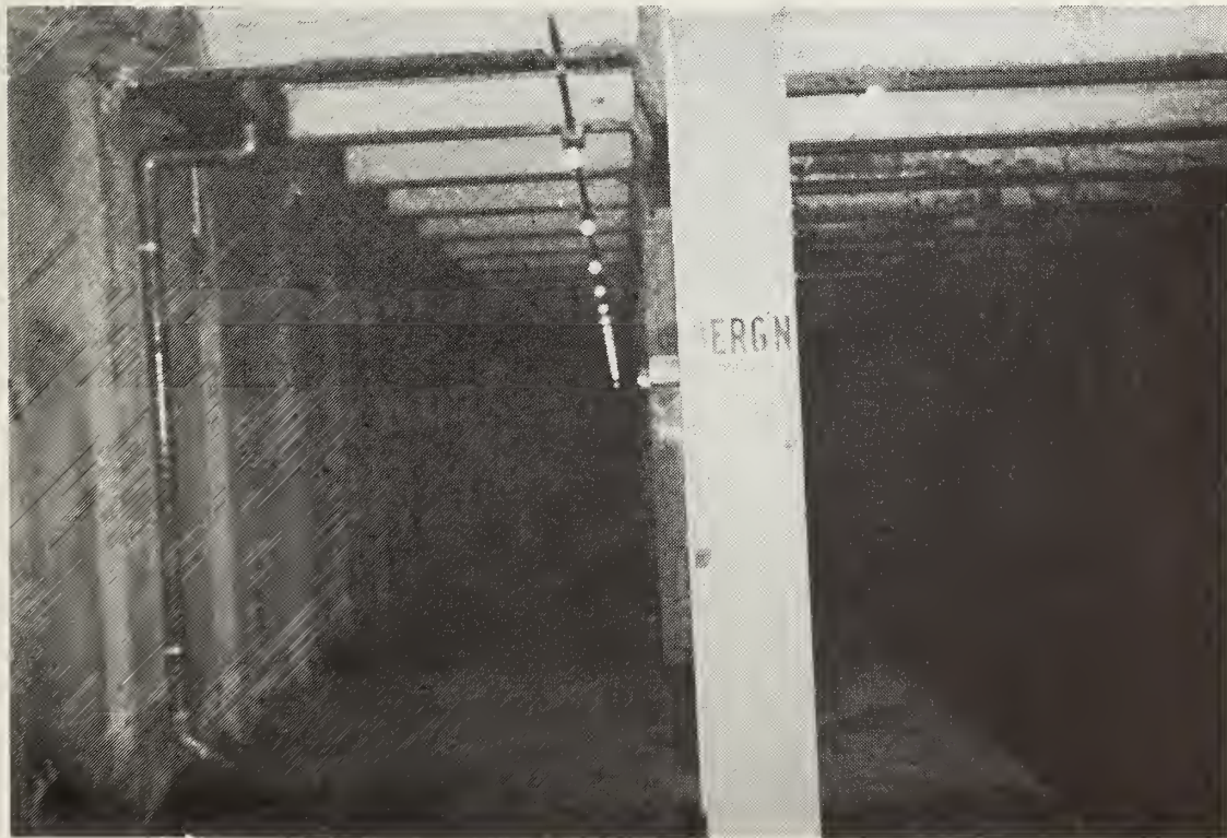
FIGURE 9.13 WATER CHANNELING (BERGEN STREET STATION)
