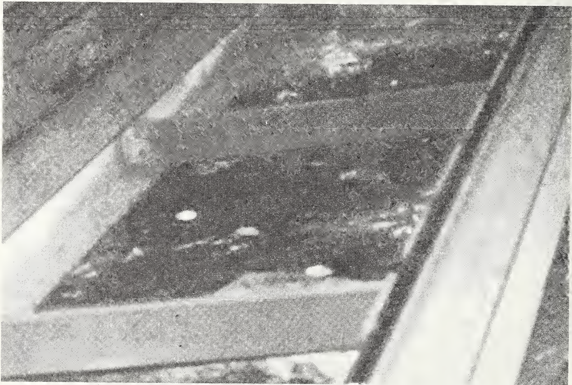
FIGURE 7.18 AREA WHERE BALLAST IS WASHED OUT COMPLETELY (ORANGE LINE, ESSEX STATION)
