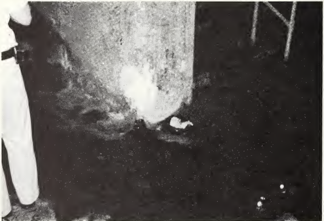
FIGURE 9.5 WATER INFILTRATION (BERGEN STREET STATION)
