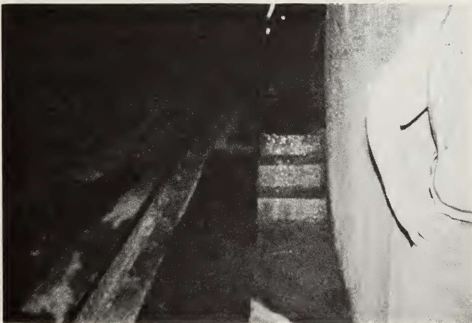
FIGURE 8.2 WATER LEAKS ON RAIL SUPERSTRUCTURE
