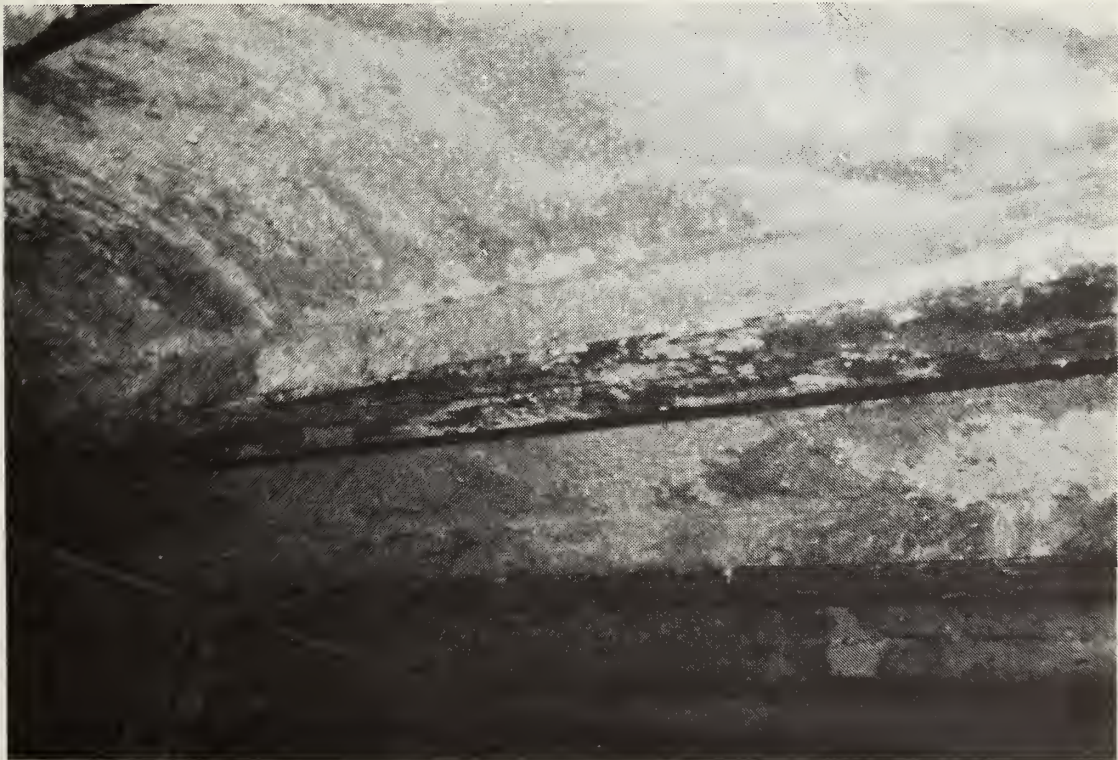
FIGURE 9.11 CORROSION OF ARCH BEAMS (BERGEN STREET STATION)
