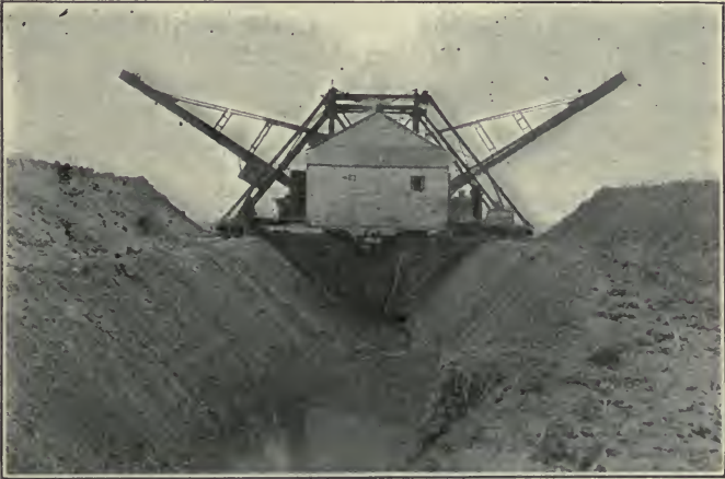
Fig. 67. An excavator for digging open ditches, which is carried on tracks laid at each side of the ditch.
