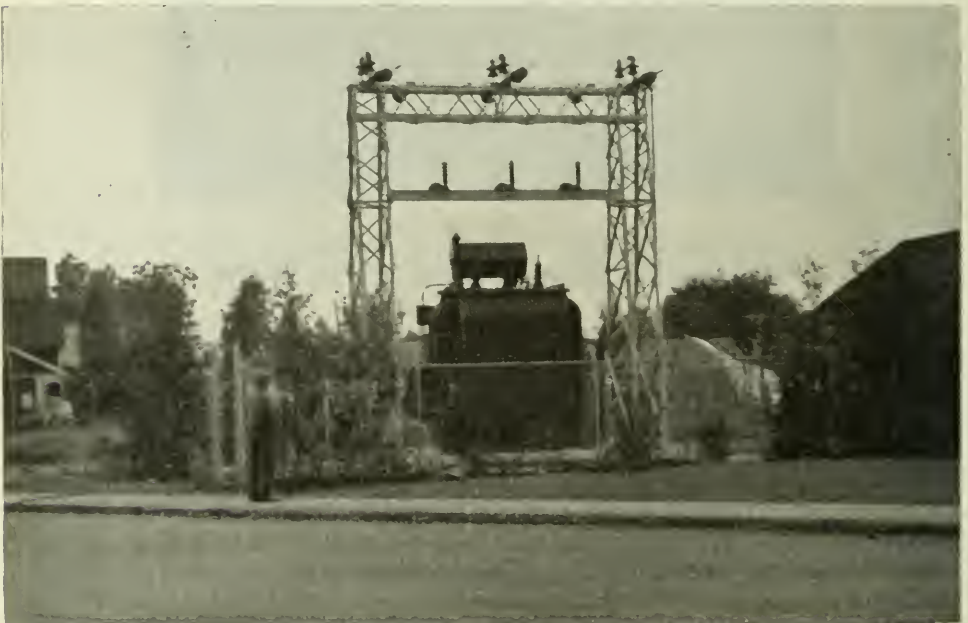
DISTRIBUTION STATION NO. 3 — EAST YORK A unit type station with site improvements
