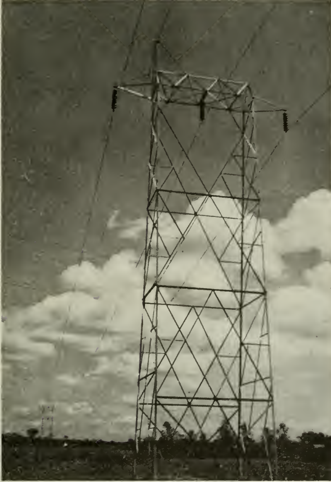
TRANSMISSION LINES — EASTERN ONTARIO SYSTEM Standard tower on 110,000-volt line from Frontenac to Sidney
