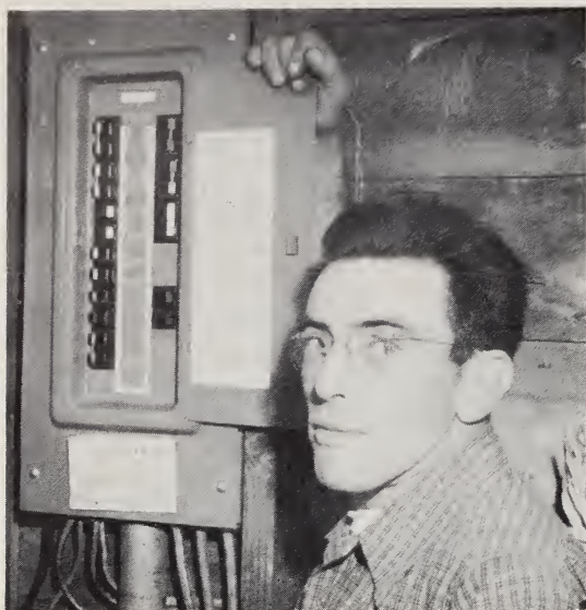
Consumer Pat Cahill won the first of forty 200-amp panels given by West Oregon Electric Co-op, Vernonia, in an 8-month re-wiring or new home offer.
