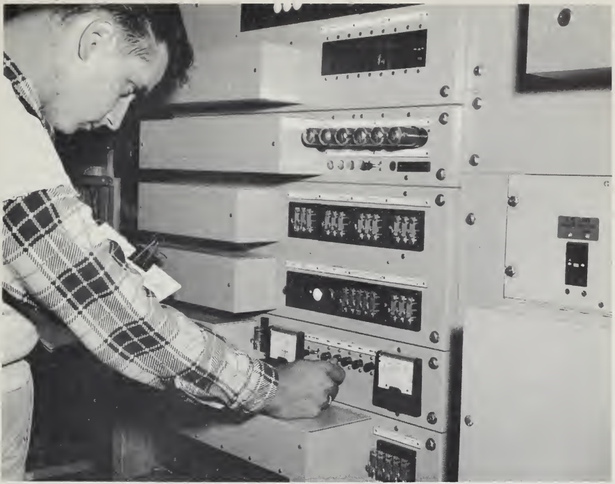
After reading meters, maintenance man makes tests.
