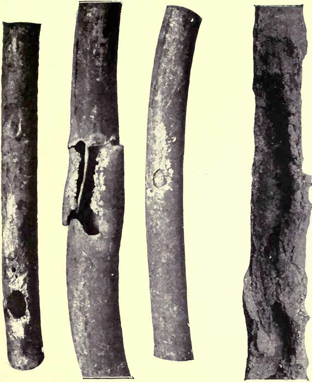
PIPE DESTROYED BY ELECTROLYTIC ACTION.
