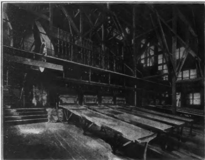
BATTERY FLOOR, CENTRAL MILL, SHOWING STEEL FRAMES, CONCRETE MORTAR BLOCKS AND BINS
