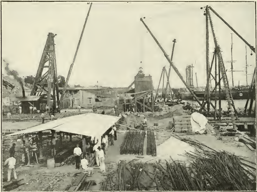
Construction work in Cuba. Plant of Snare & Triest at Casa Blanca on Havana Harbor for making reinforced concrete piles.
