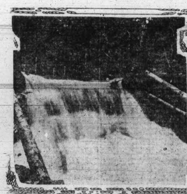
WEIR NO. 3, ON EAST BRANCH OF MILLSTREAM This Photo Was Taken Just Below the Main Point of Storage, When the Water Was Running at the Rate of Twenty-Nine Million Gallons Per Day.
