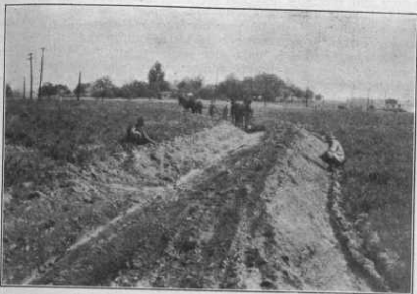
FIGURE 19.—Terrace construction with the plow and V-drag. It requires considerable work to develop satisfactory terraces with this type of equipment.
