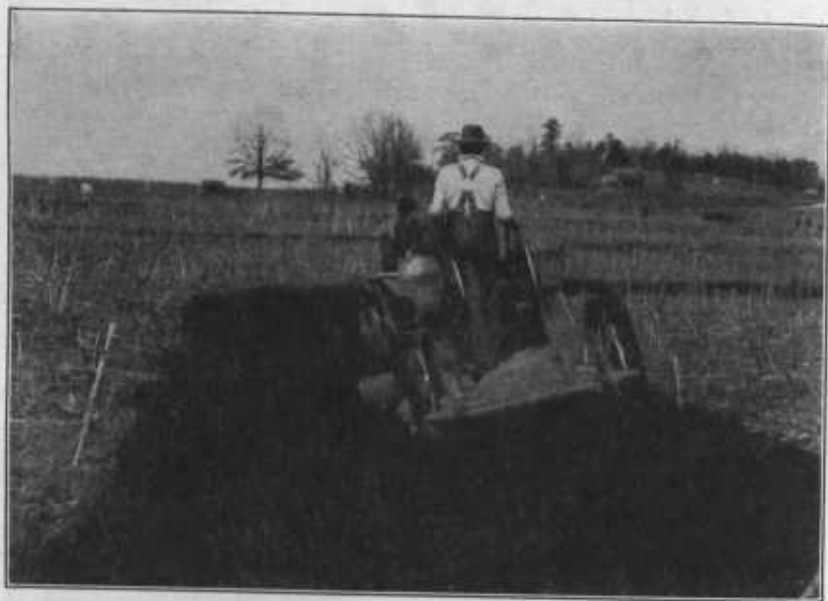
FIGURE 21.—Terracing with a 10-foot blade terracer and crawler-type tractor. This type of equipment is used extensively for terrace construction.
