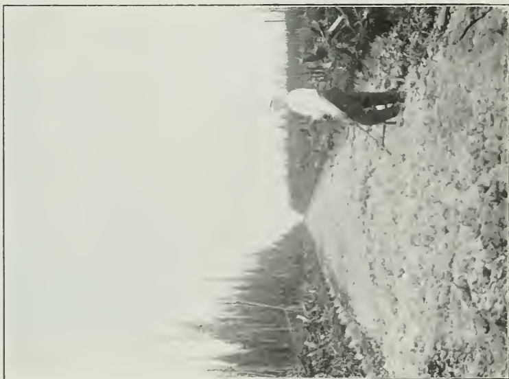
New road on the boundary between the Townships of Armstrong and Evanturel
