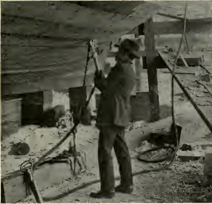
Fig. 99. The Caulking Tool Can Be Held in Any Position and Is Able to Deliver 1,500 Taps a Minute. The Oakum Is Fed Mechanically, so That The Work of "Horsing It In" Can Be Done Rapidly and Thoroughly, No Matter Where the Seam Is Located
