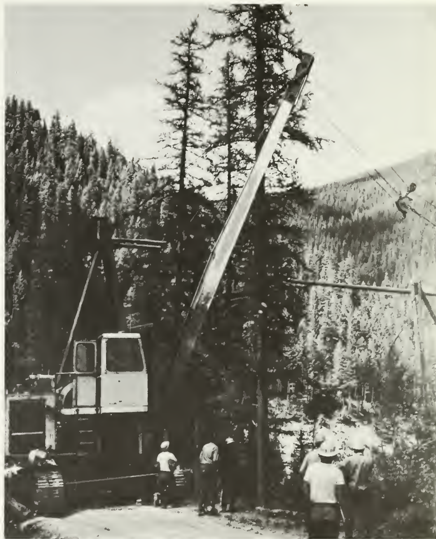
Researchers are investigating the environmental and management consequences of carrying out intensive wood fiber utilization with methods such as this skyline yarding system.
