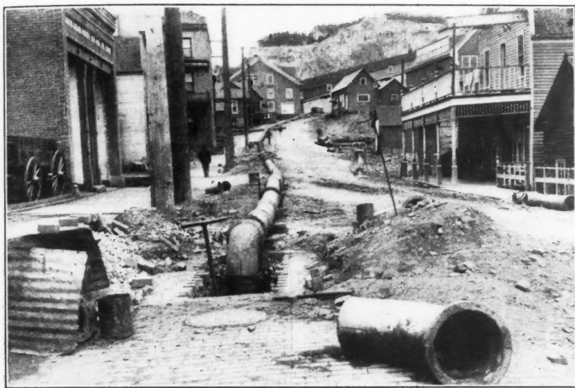
TEMPORARY PIPE FROM CITY MAINS TO THE OPEN CUT OF THE HOMESTAKE MINE
