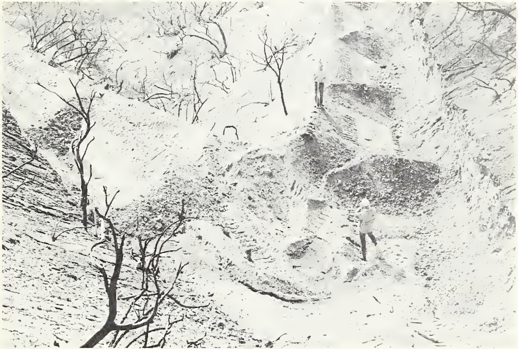
Figure 8.--Completed trench. The basins hold runoff and lessen the lateral movement of water within the trench.
