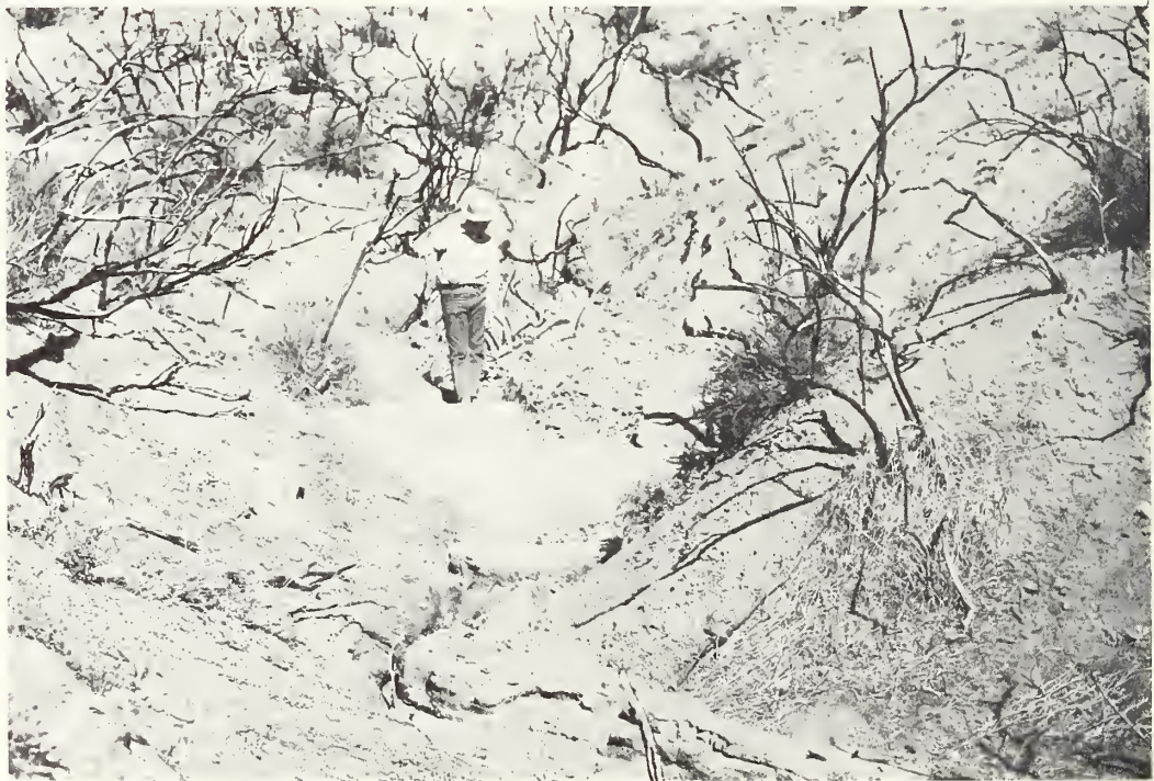
Figure 9.--Stream channel checks. Their purpose is to prevent channel downcutting and to stabilize canyon side slopes.
