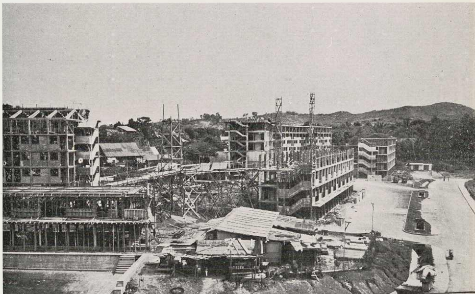
Flats under construction in Kampong Tiong Bahru Fire Site. The building at the far end is provided with a clinic on the ground floor.
