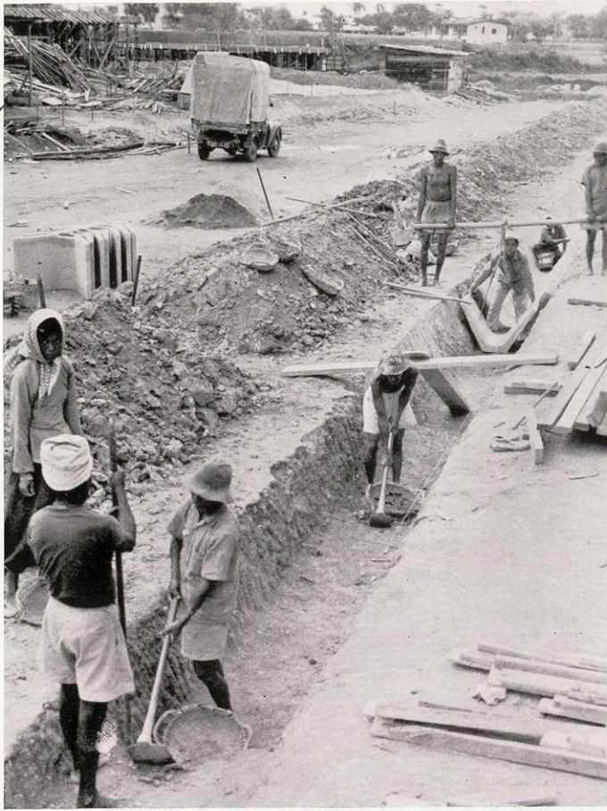
Construction and laying of roadside drains for Housing and Development Board Estates
