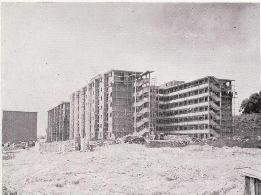
Duchess Estate Contract 7 Phase II. Comprising 4 and 7 storey flats of 2 and 3 room units (under construction)
