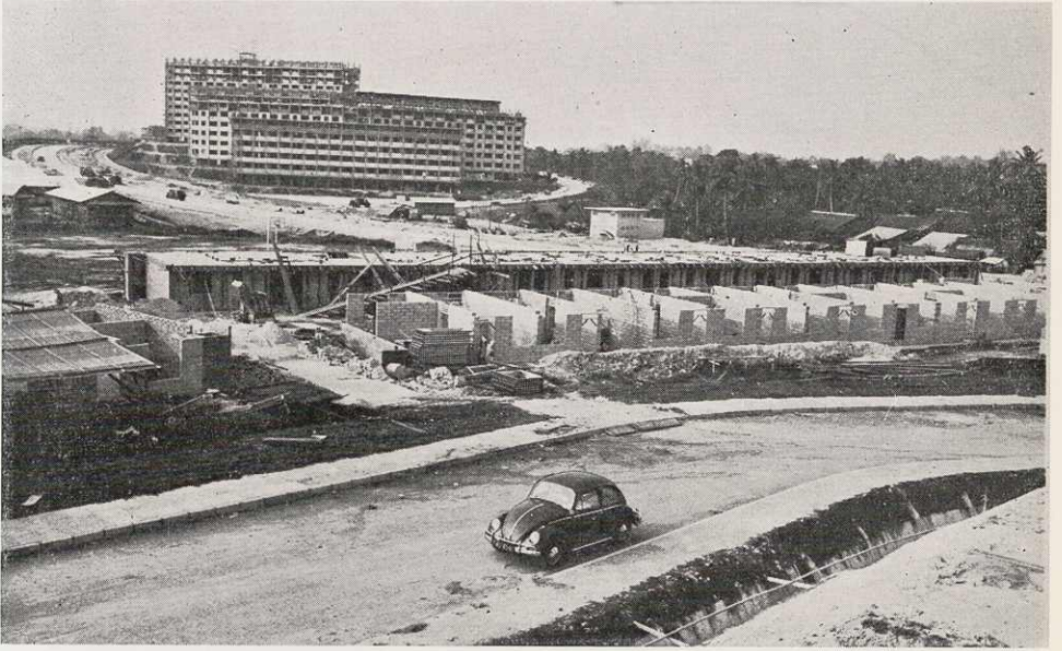
A general view of the 2-storey terrace houses under construction in Neighbourhood V, Queenstown.
