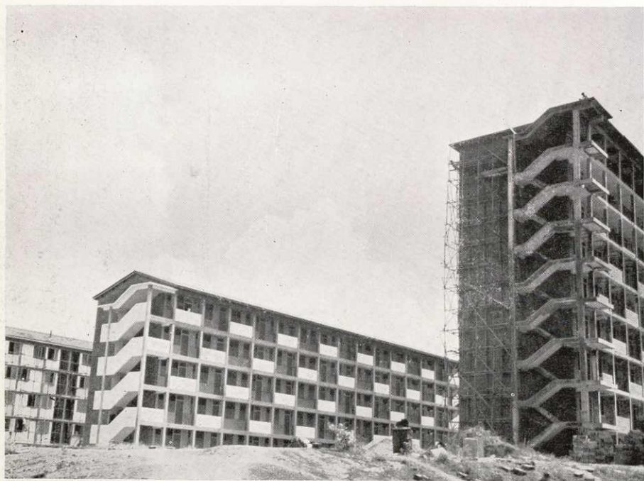
Kampong Tiong Bahru Fire Site Phase III, 5 and 9 storey 2 room units with shopping facilities at ground floor under construction
