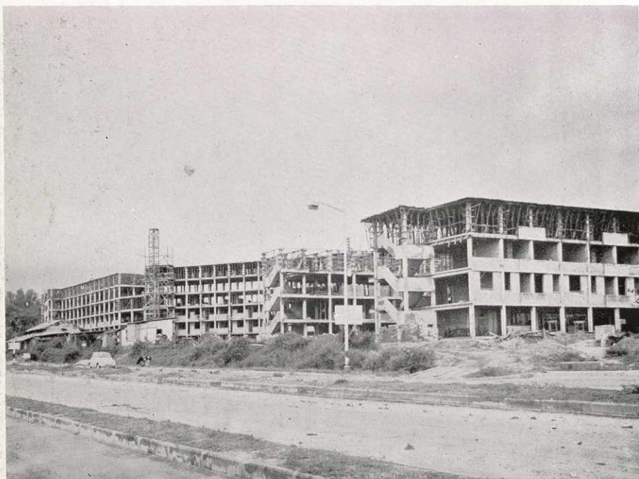
Duchess Estate Contract 7 Phase I. Comprising 4 and 7 storey flats of 1, 2 and 3 room units with shopping facilities at ground floor (under construction)
