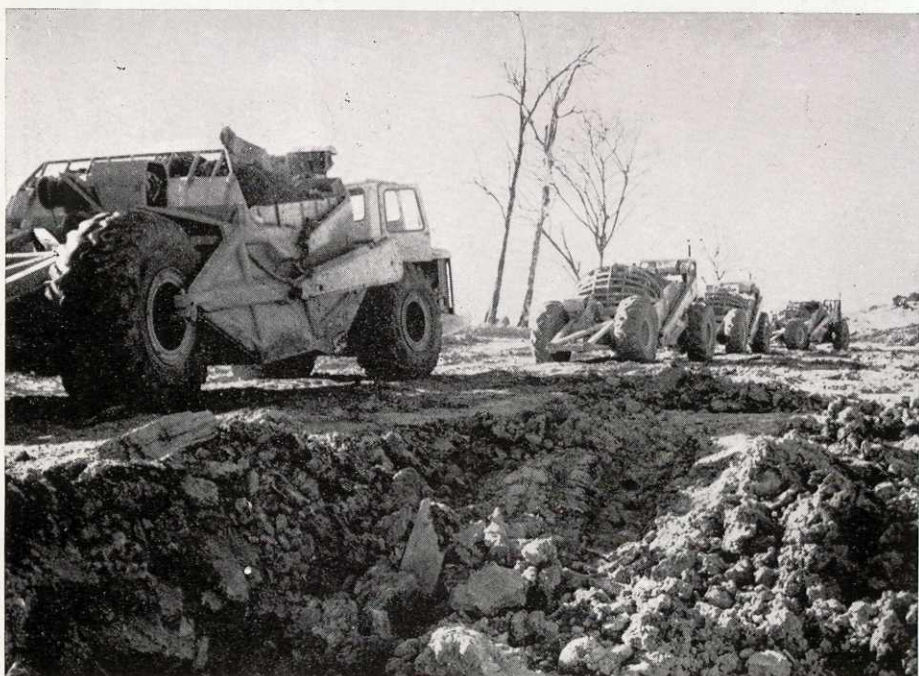
The Board's earthmoving machinery fleet in operation on levelling of platforms for Queenstown Neighbourhood IV
