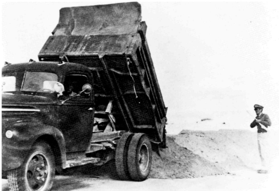
Figure 12. Pouring gypsum for road shoulder construction (1930s). Courtesy White Sands National Monument.
