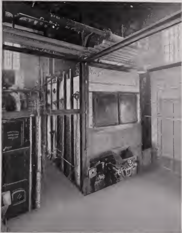
400 H. P. FREEMAN WATER TUBE BOILER
