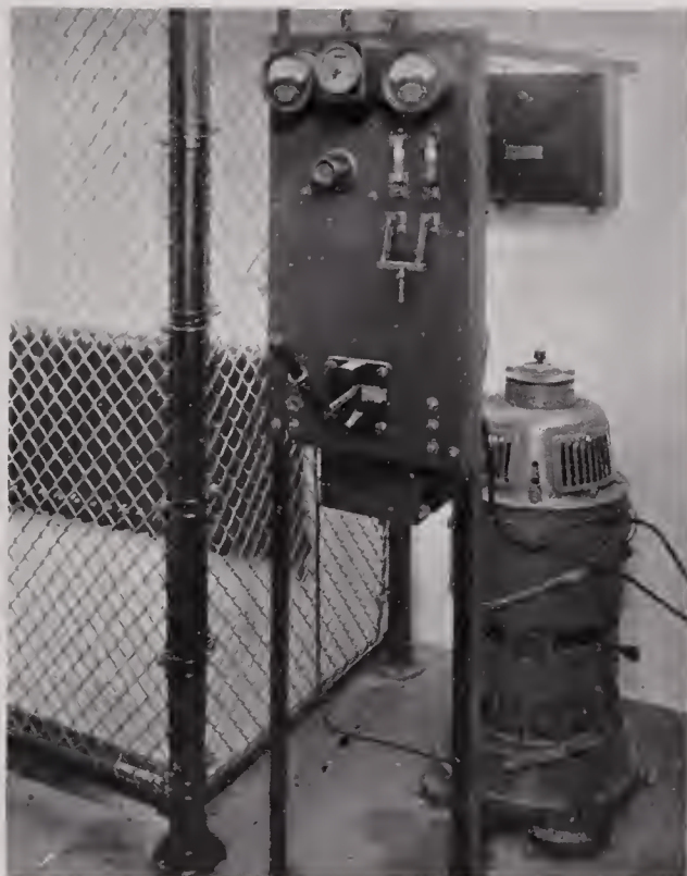
BATTERY CHARGING GENERATOR
