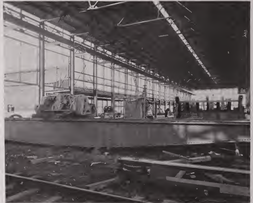
10-TON CRANE FOR WAREHOUSE This is a Duplicate of the Hammer Shop Crane
