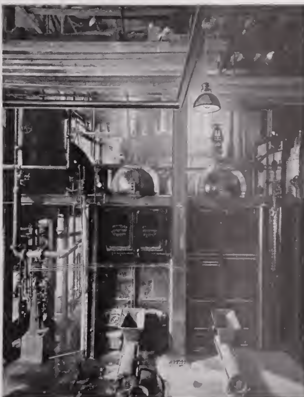
TWO 150 H. P. FRANKLIN BOILERS
