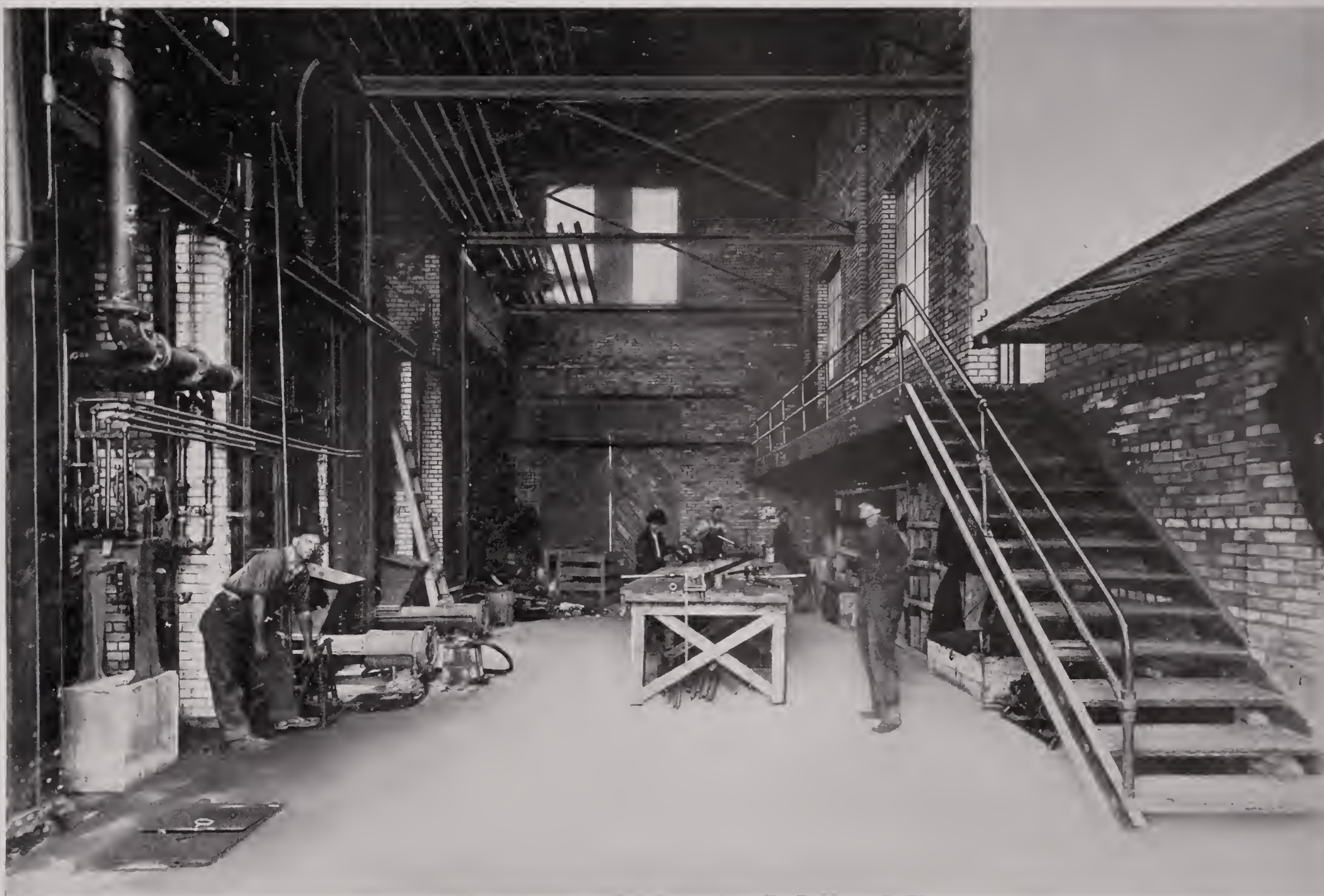
THE BOILER ROOM IN MAIN POWER PLANT
