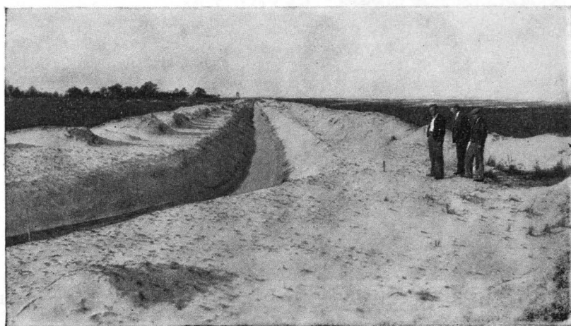
FIGURE 46.—Main drainage ditch through sandy soil, Cat Island, Miss., dug by C. W. A. workers as a mosquito-control measure.
