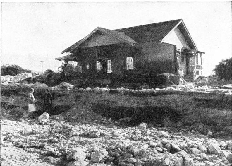
FIGURE 32.—This Montrose cottage is one of the 400 homes wrecked by the New Year's flood from the fire denuded watershed. The great gully in foreground carried away lawn and garden.
