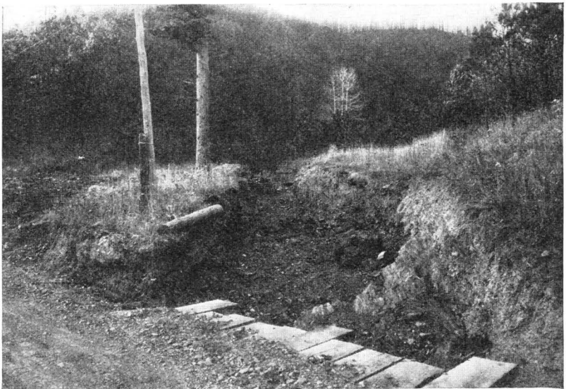
FIGURE 22.—Another view of the gully shown in figure 21. An 18-inch culvert was adequate before the drainage basin was burned over.
