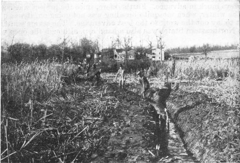
FIGURE 47.—C. W. A. workers clearing, straightening, and deepening stream through marsh at Westminster, Md., in carrying out mosquito-control project.
