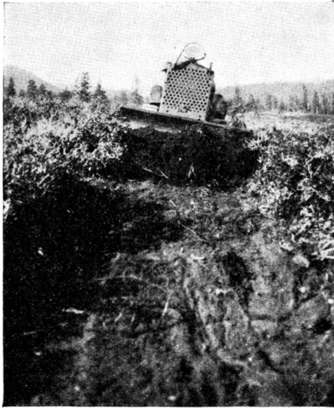
FIGURE 13.—The tractor pushes up a pile of dirt as it completes the clearing of a strip.
