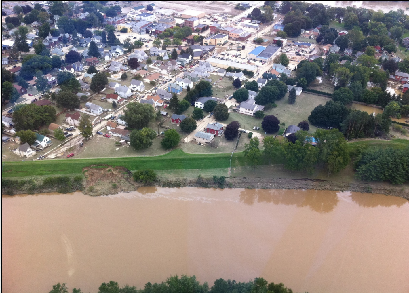
Athens – Chemung River, PA – Damage to Levee
