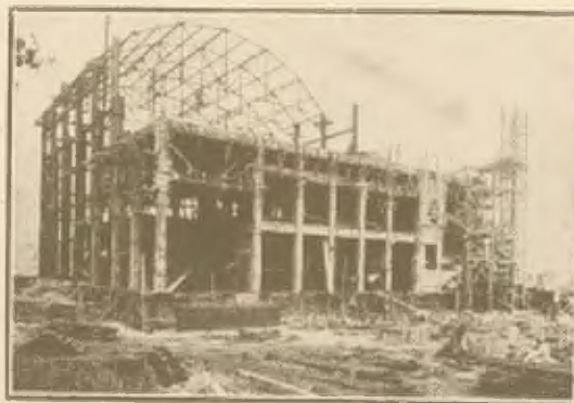
CHAPEI POWER PLANT, SHANGHAI.
