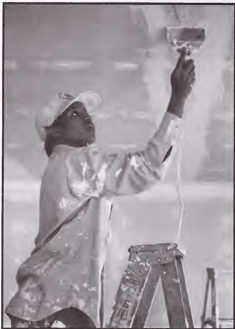
A Job Corps student puts up drywall in a building to be used for the Head Start Program.
