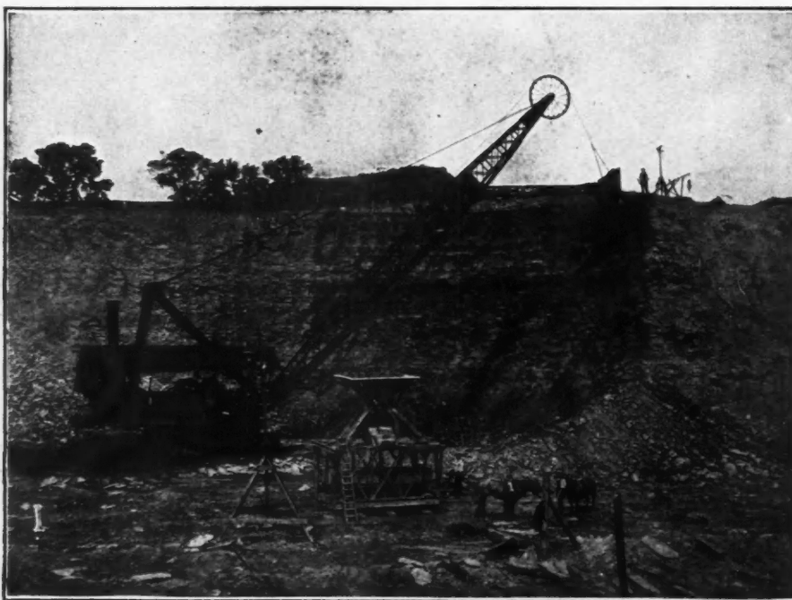
GIANT EXCAVATOR MAKING 60-FOOT CUT—TWO CARS LOADED SIMULTANEOUSLY THROUGH HOPPER IN FOREGROUND
