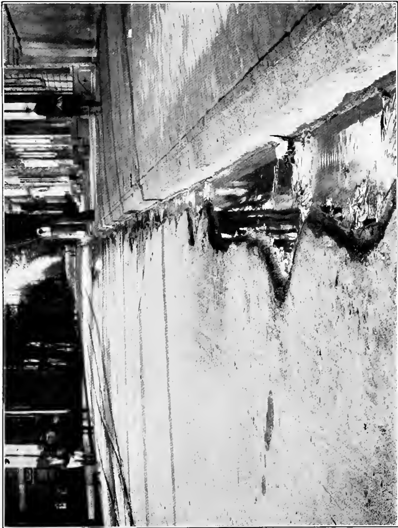
FIG. 27.—Bermudez Asphalt Surface Disintegrated by Water.
