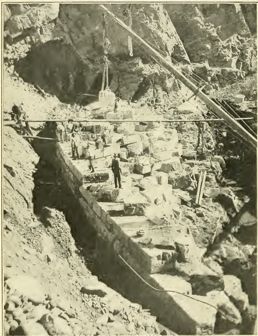
LAYING FOUNDATION OF ROOSEVELT DAM. Foundation covers more than an acre of ground.
