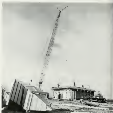
Tower frames are placed on roof of station building for TD-3 microwave system trial.
