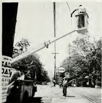
A Bell Company puts up coaxial cable for channel service provided to CATV operator.
