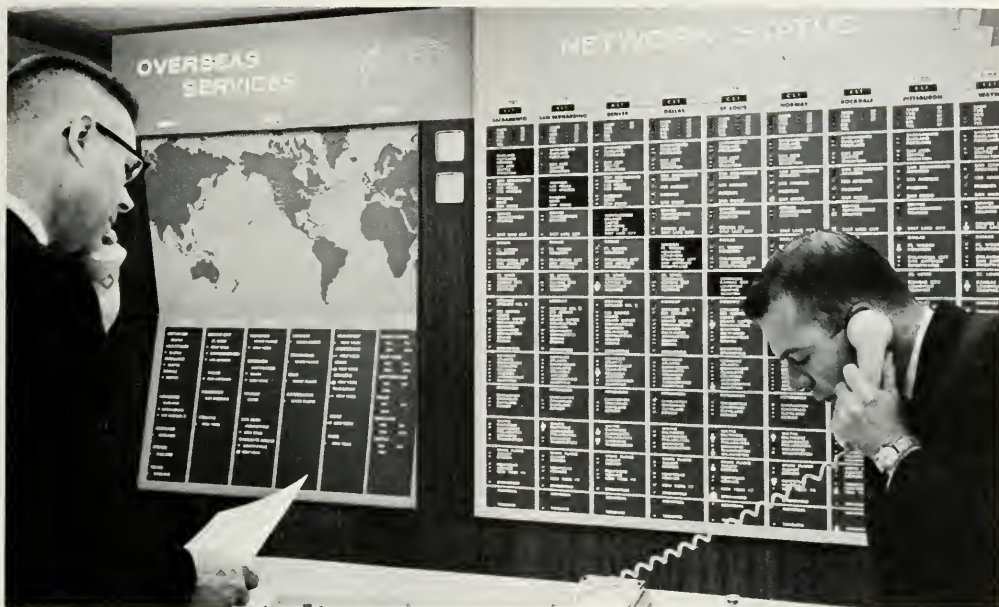
Network management centers keep tabs on calling volumes and equipment irregularities so alternate routes can be quickly estab-
