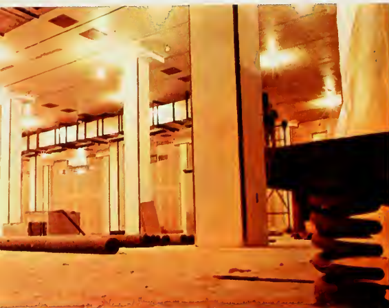
All communications and ventilating equipment is protected from damage by mounting it on coil springs and rubber cushions.
