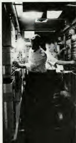
In this central office at Suitland, C. & P. Tel. Co. Plant men are on 24-hour duty to insure continuous quality performance of NESC communications system.
