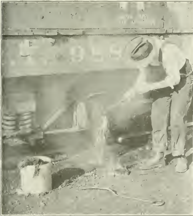
Cleaning Out a Hot Box Preparatory to the Application of Mohawk Cooling Compound
