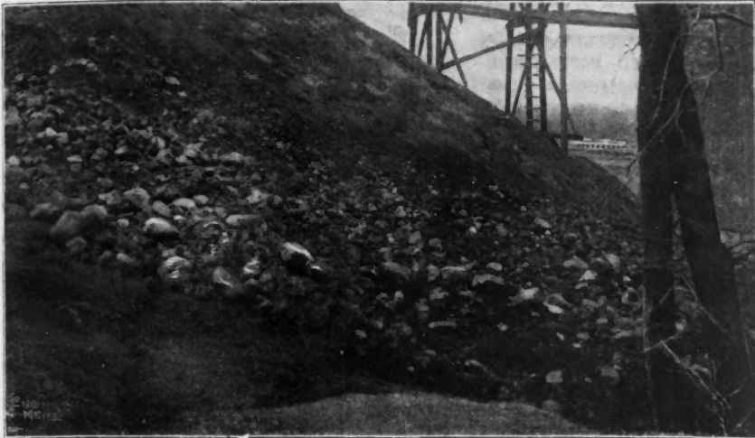
FIG. 3.—VIEW OF MATERIAL AT FOOT OF EMBANKMENT SHOWING LAVA-LIKE APPEARANCE OF FLOWING CLAY.
