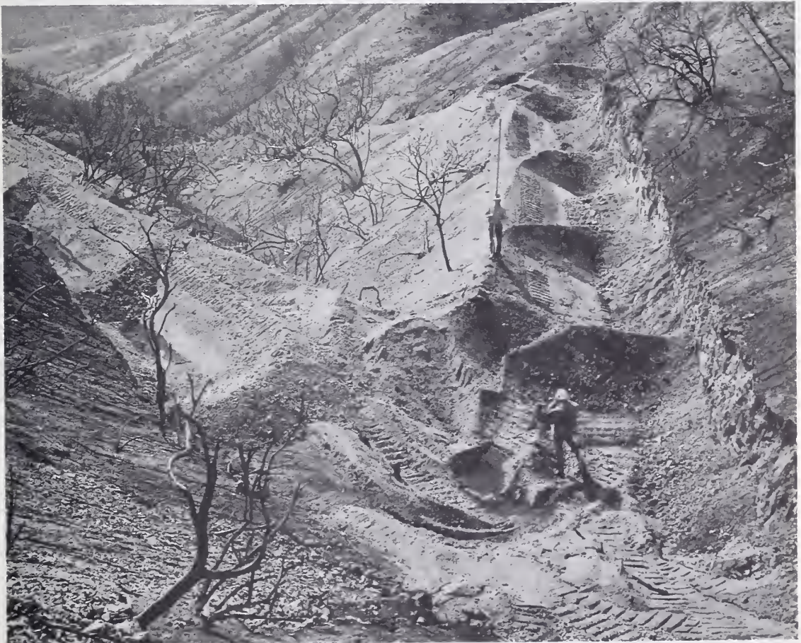
Completed terrace. The listed basins hold runoff and lessen the lateral movement of water within the terrace.
