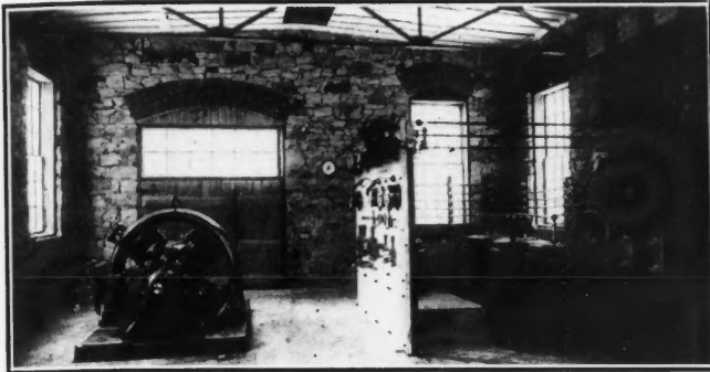
FIG. 2. INTERIOR GRAHAM SUB-STATION
