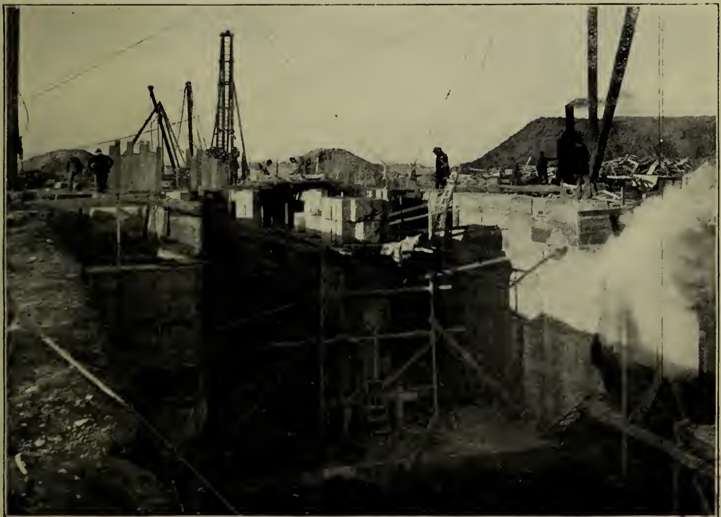
HIGH-LEVEL SEWER—SCREEN CHAMBER AND SAND CATCHER ON NUT ISLAND IN CONSTRUCTION—VIEWS FROM OPPOSITE ENDS.
