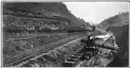
The big Cut through the Culebra Divide, showing Steam-Excavators at Work at the various Levels This cut is the highest part of the canal. When finished it will be sixty-eight feet above sea-level. The excavation is about two-thirds completed
