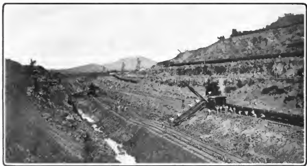
The Eastern End of the big Culebra Cut, with Steam-Excavators and Work-Trains at the various Levels
