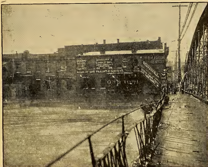
TWISTED RAILING ON STATE STREET BRIDGE
