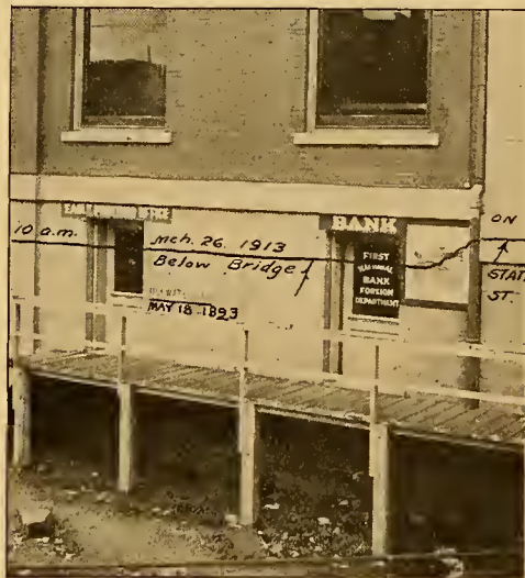
HIGH WATER MARKS AT STATE STREET BRIDGE
