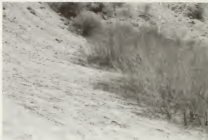
Figure 4.—This buffer strip of willows developed naturally at the toe of a cut slope. About 40 years ago, the slope was created by the excavation of borrow material near Anderson Ranch Reservoir in the Idaho batholith. Note the concave shape of the slope's toe that was formed of colluvial material by the buffer strip.
