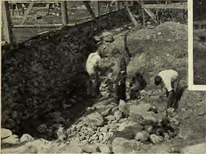
Laying the cellar wall. More than 20 tons of concrete and 150 tons of rock and gravel went into the foundation. All the work of hauling and mixing was done by the older club boys.
