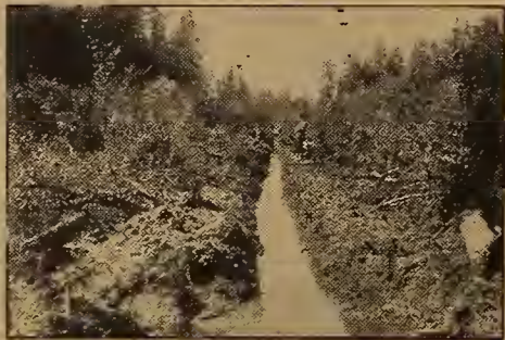
This ditch was blasted through thick underbrush filled with stumps, roots, and logs
