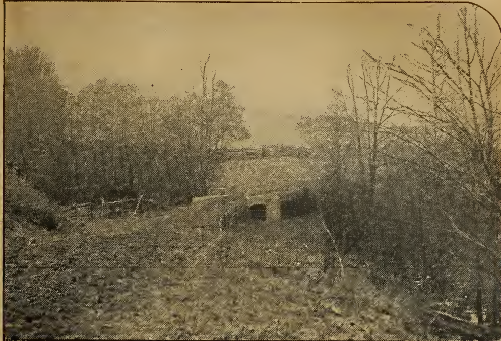
THIS well-constructed, reinforced concrete bridge replaced a wooden structure that had done service for many years. The difference in repairs and the permanence of the concrete bridge were the factors in its favor. The earth road in the foreground has been graded and crowned. The next step will be to roll it with a steam roller or a large horse-drawn roller.
