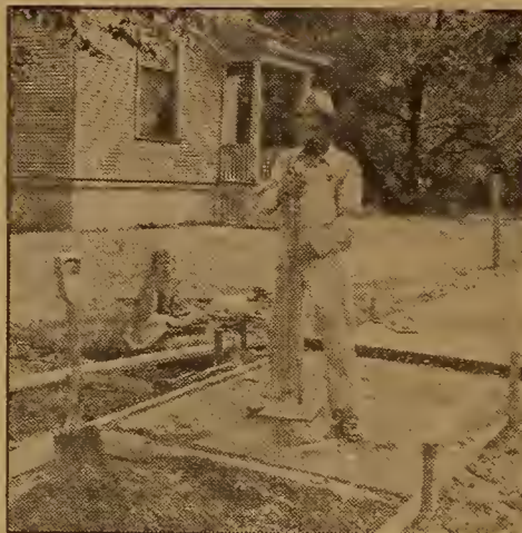
The concrete is heaped in the form, and is tamped to grade. The grade is the top of the 2x4's
