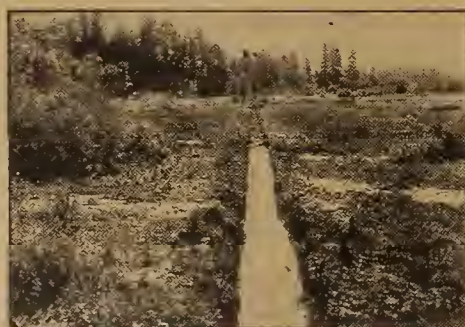
This portion of the ditch is through a swamp. Four men blasted 600 feet in two hours
