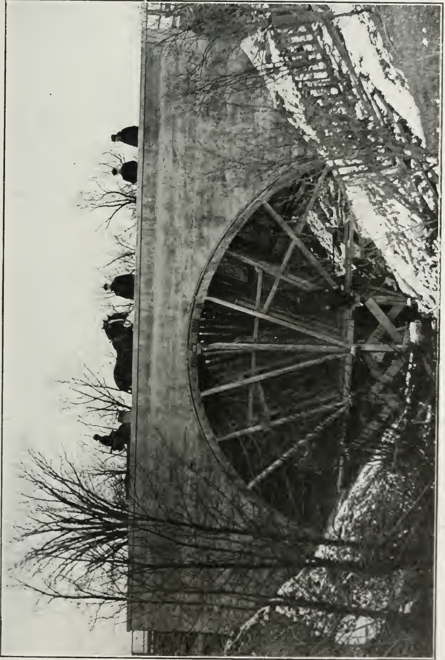
A Peel County Concrete Arch, near Cooksville. The arch, with timber centering in place, is on Dundas Street, and has a rise of 17 feet and a span of 40 feet.
