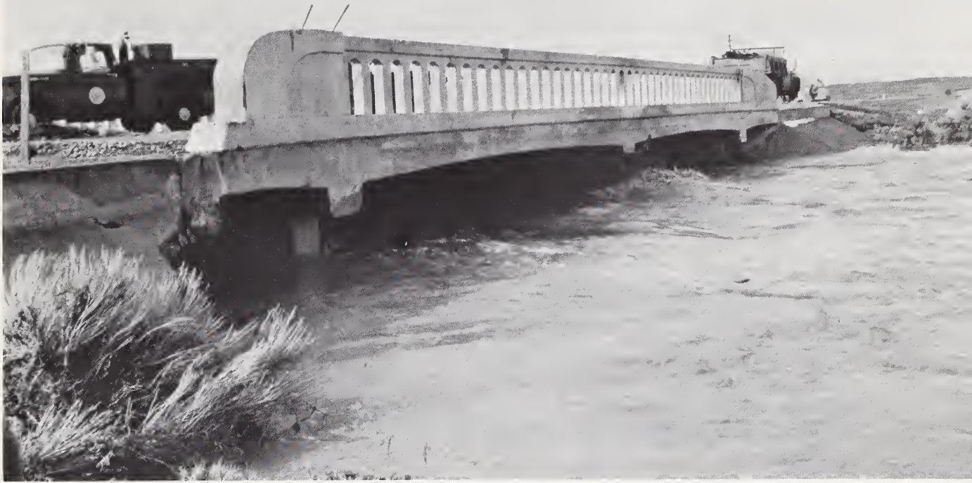
Photograph 6. - Closeup of underside of North Fork Bridge, February 13, 1962, showing North Fork high waters and damage to bridge abutment on left side of photograph. Looking west.
