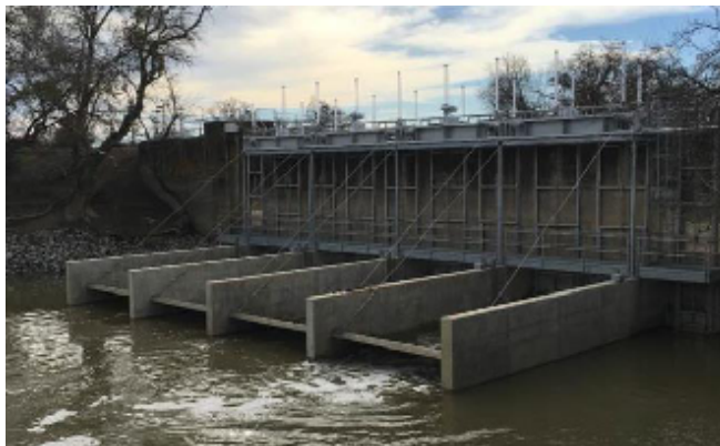
Fig. 6. Knights Landing Outfall Gates (KLOG)
