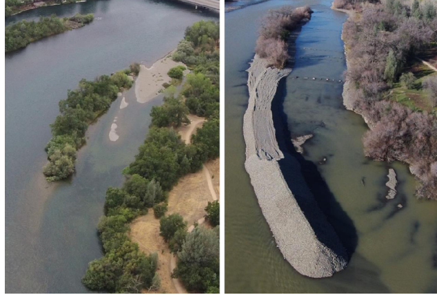
Fig. 5. 2015 Diversions Painters Riffle Restoration Project completed by GCID. Video can be seen at http://www.gcid.net/#!painters-riffle-project/qs7o8
