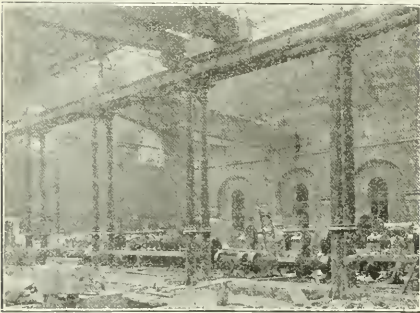
EDINBURGH: TOLL-CROSS CABLE POWER, INTERIOR OF ENGINE-ROOM (ENGINES IN COURSE OF ERECTION).
