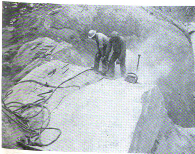
Miles of hose and pipe are used to carry the compressed air which operates dozens of pneumatic drills. The jack hammer, shown operating without dust control, drills 2-inch holes 11 inches per minute in hard granite. Wet drilling eliminates this dust exposure.
