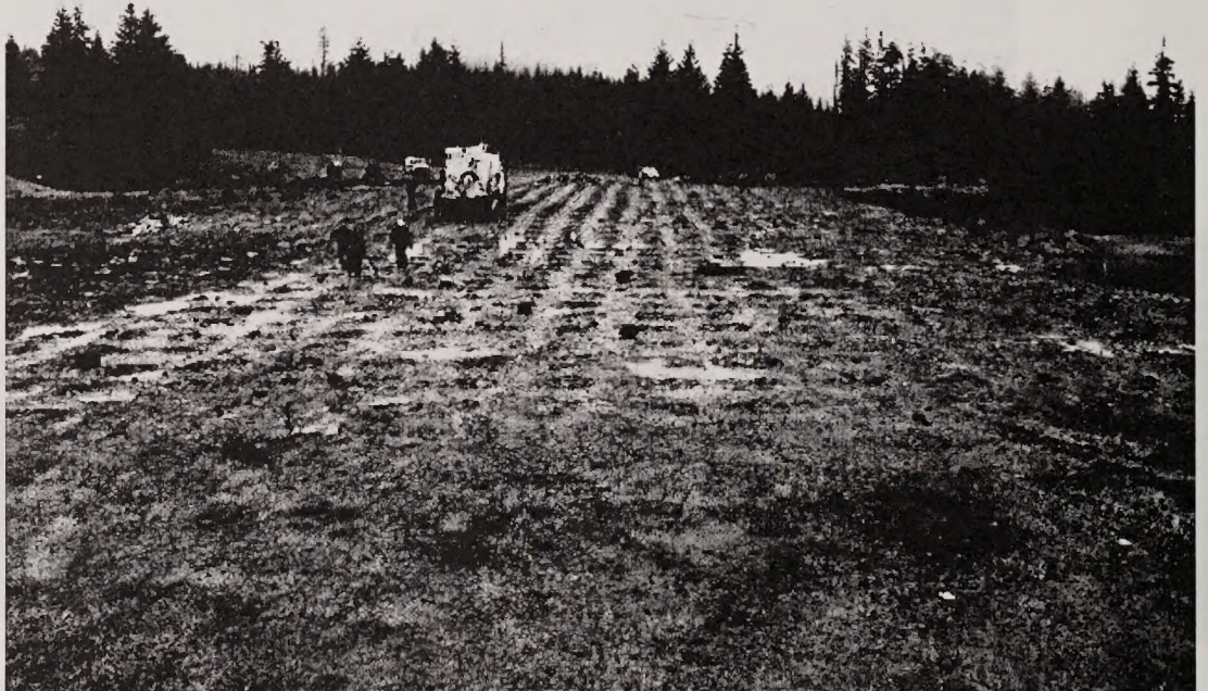
Packing drill holes with explosives at Elk Wallow Quarry before the 'shot'
