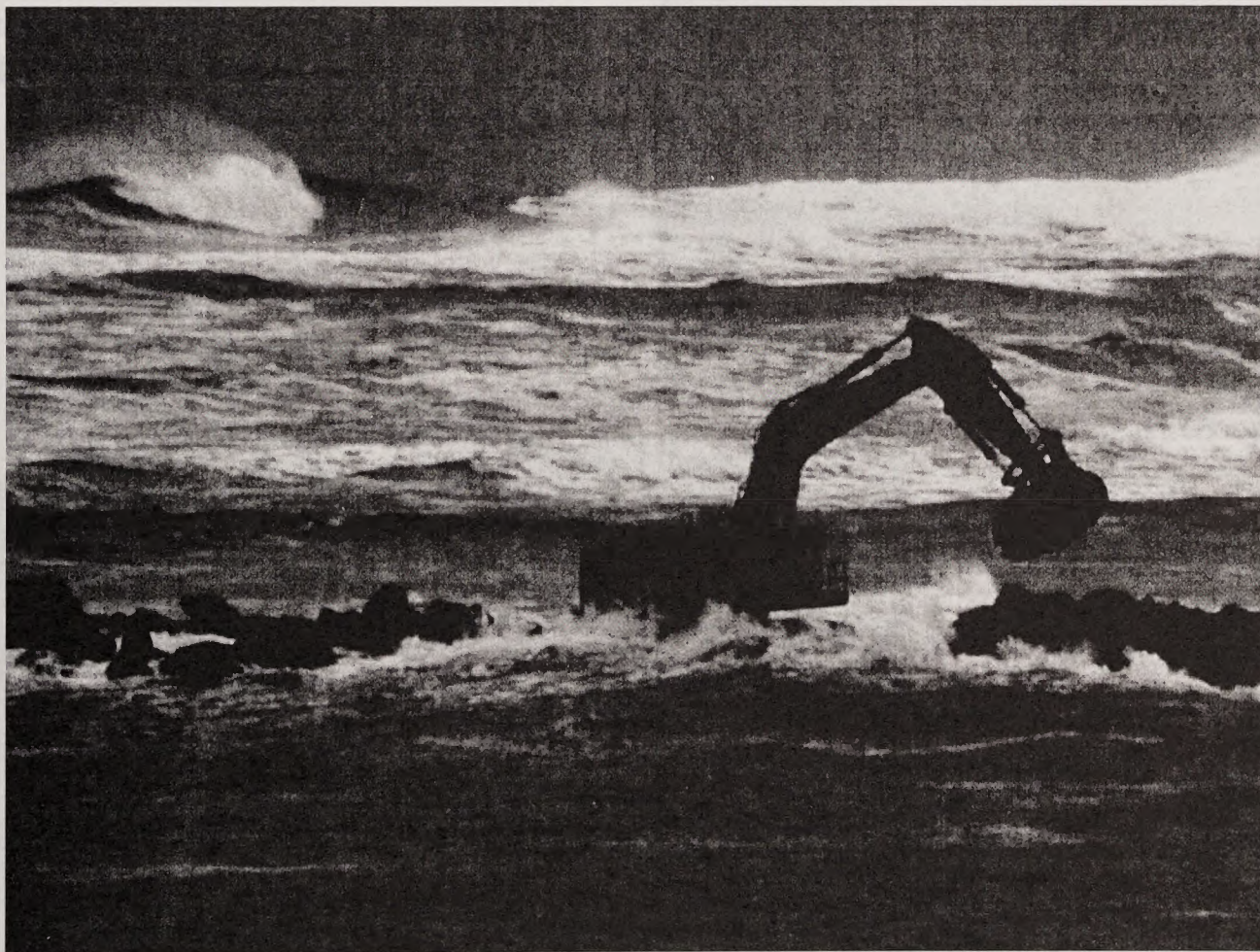
Access through BLM lands allows adjacent landowners to manage their lands - such as the Corps of Engineers conducting emergency repair to the North Jetty of Coos Bay
