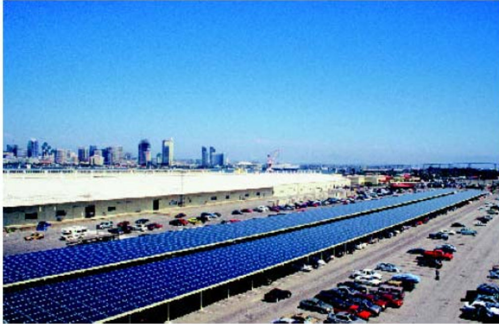
Figure 3. PV System at Coronado Base, CA
