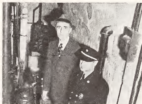
Many fires originate in basements and furnace rooms. Here Mr. Coulter inspects the Byrd furnace room with a fire official.
