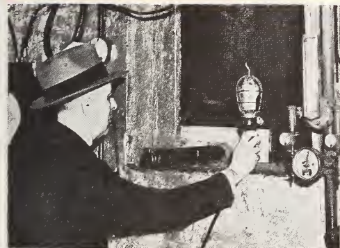
Manager Robert Coulter of the Byrd theatre in Richmond, Va., inspecting air ducts for trash. Fire spreads easily through air ducts.
