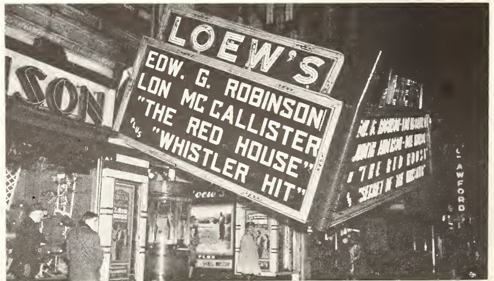
THE HIT HOUSE —hit by a 60-mile-an-hour gale, March 24, in Indianapolis. The marquee sank to within five feet of the sidewalk.
