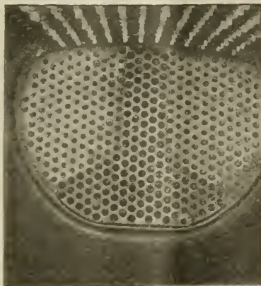
FIRE BOX END OF LOCOMOTIVE BOILER TUBES PARTIALLY WELDED. LIGHT AREAS SHOW WELDED TUBES AND DARK AREA SHOWS TUBES READY FOR WELDING.
