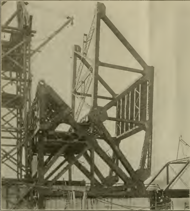
C & N. W. RY. DEERING BRIDGE—FIRST STAGE OF ERECTION. THE COUNTERWEIGHT PIVOT AND BASCULE SPAN PLACED READY FOR PERMANENT SETTING.
