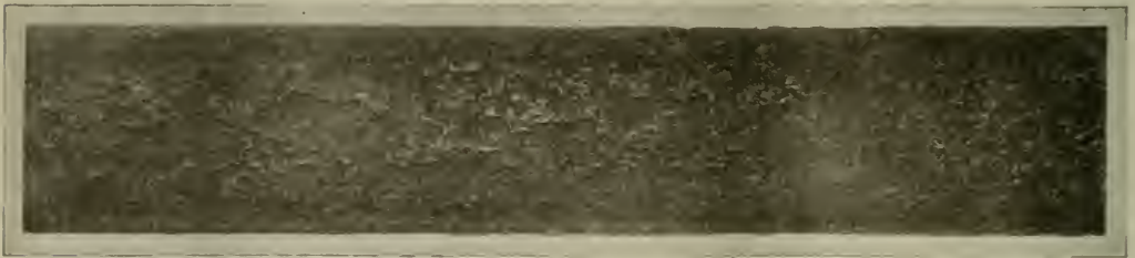
WROUGHT IRON PIPE AFTER IMMERSION IN RUNNING MINE WATER. COMPARATIVE LOSS BY CORROSION: SPELLERIZED STEEL PIPE, 73 PER CENT; WROUGHT IRON, 100 PER CENT.
