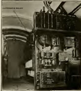
INTERIOR OF CAB SHOWING MAIN SWITCH
