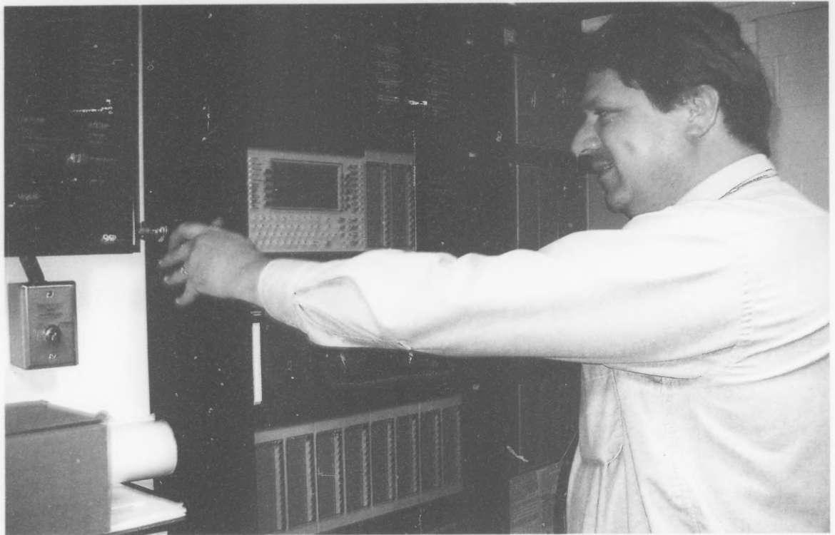
Building Management Specialist Jim Frazier checks the fire alarm board.
