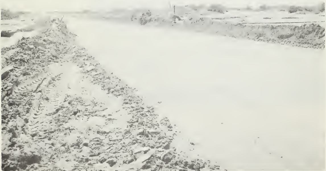
Highway 54 road damage Note sediment deposition.
