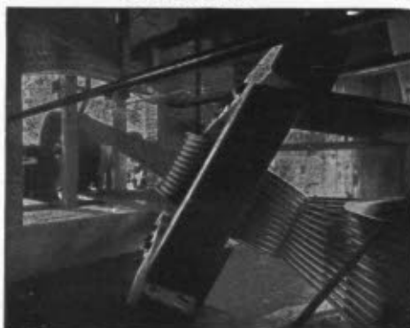
View of 500 H.P. Quarter-Twist, American System Rope Drive, from vertical water wheel shaft to Jack-shaft in generator room, Electric Light Station, Pillsbury-Washburn Flour Mills Co., Minneapolis. Installed 1900.
